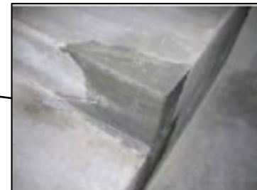
Condition at joint between old and new concrete
