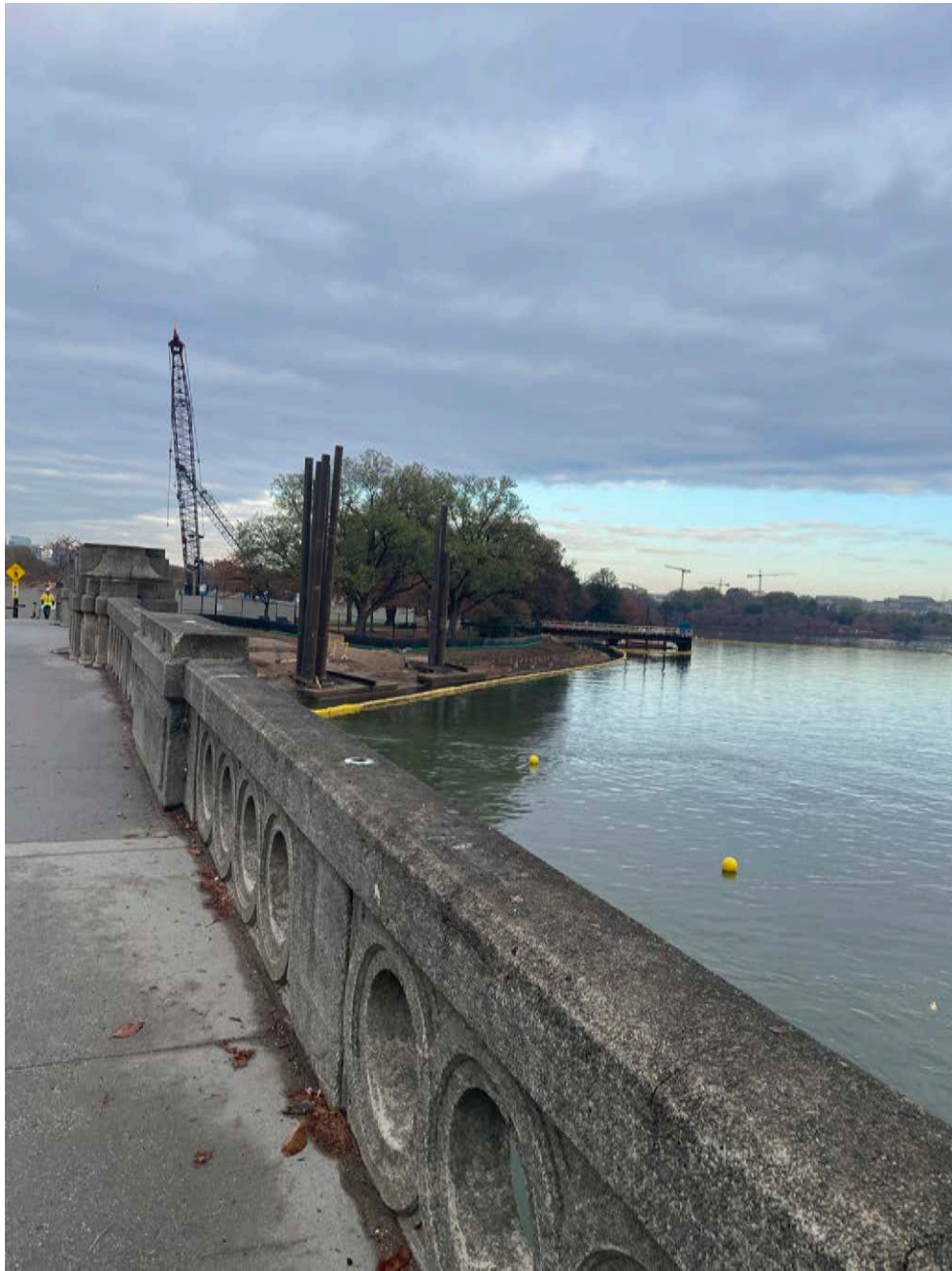
Image shows construction at the seawall north of the inlet bridge. Inlet bridge in the foreground. Crane, piling, and sediment control seen in the background.
