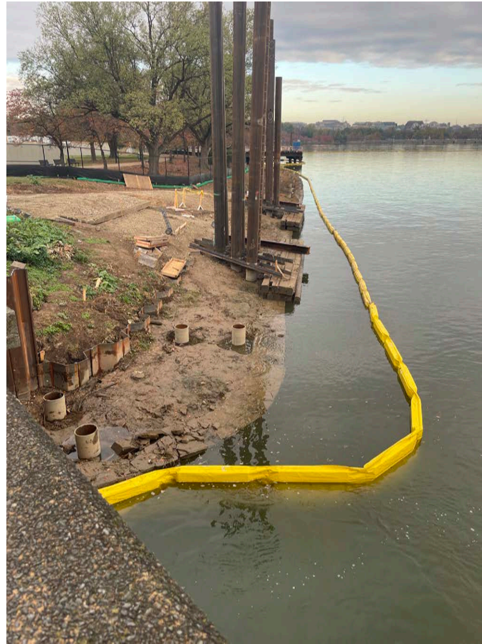
Image shows close up of construction at the seawall north of the inlet bridge. Piling and sediment control seen in the foreground. Water level has inundated the existing wall elevation.
