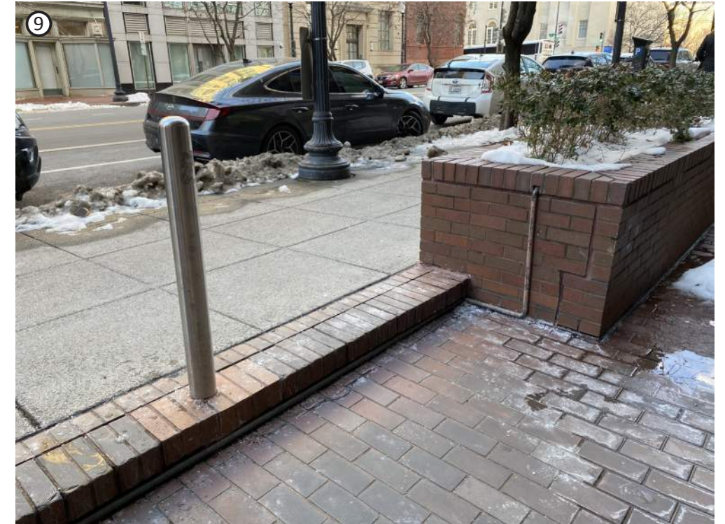
9 BOLLARDS PREVENT VEHICLES FROM ENTERING THE SITE. A SINGLE RISER CREATES A TRIPPING HAZARD
