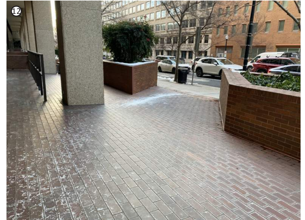
12 EXCESSIVE USE OF BRICK BLENDS WITH THE HISTORIC DISTRICT AESTHETIC, BUT CAN CONTRIBUTE TO EXCESSIVE ENVIRONMENTAL HEAT ESPECIALLY IN THE SUMMER
