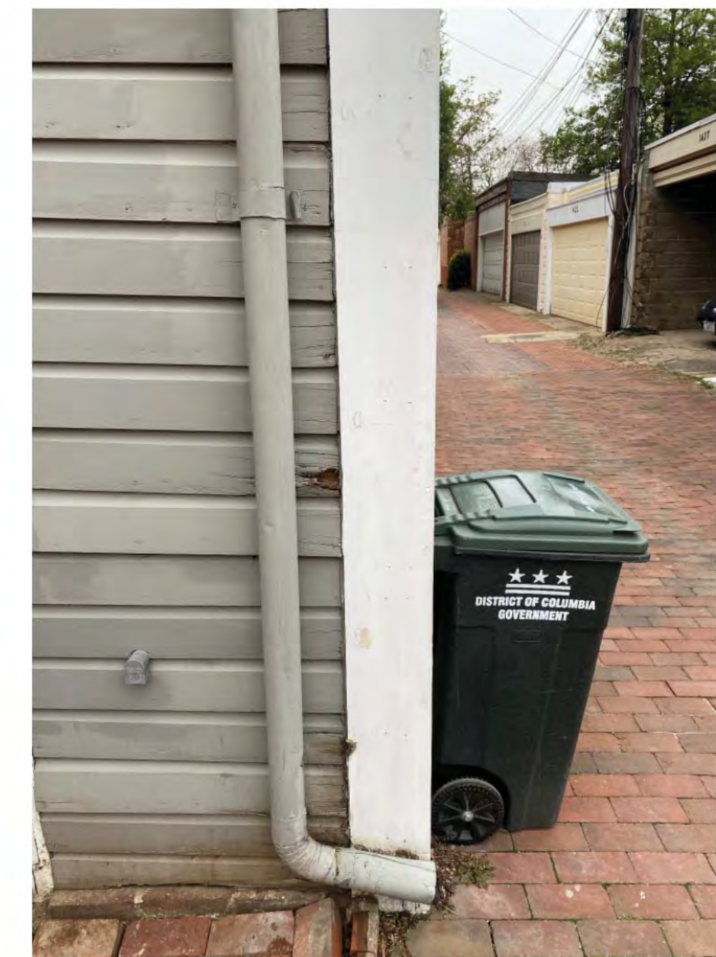
NORTH WEST CORNER SHOWING SIDING ROT
