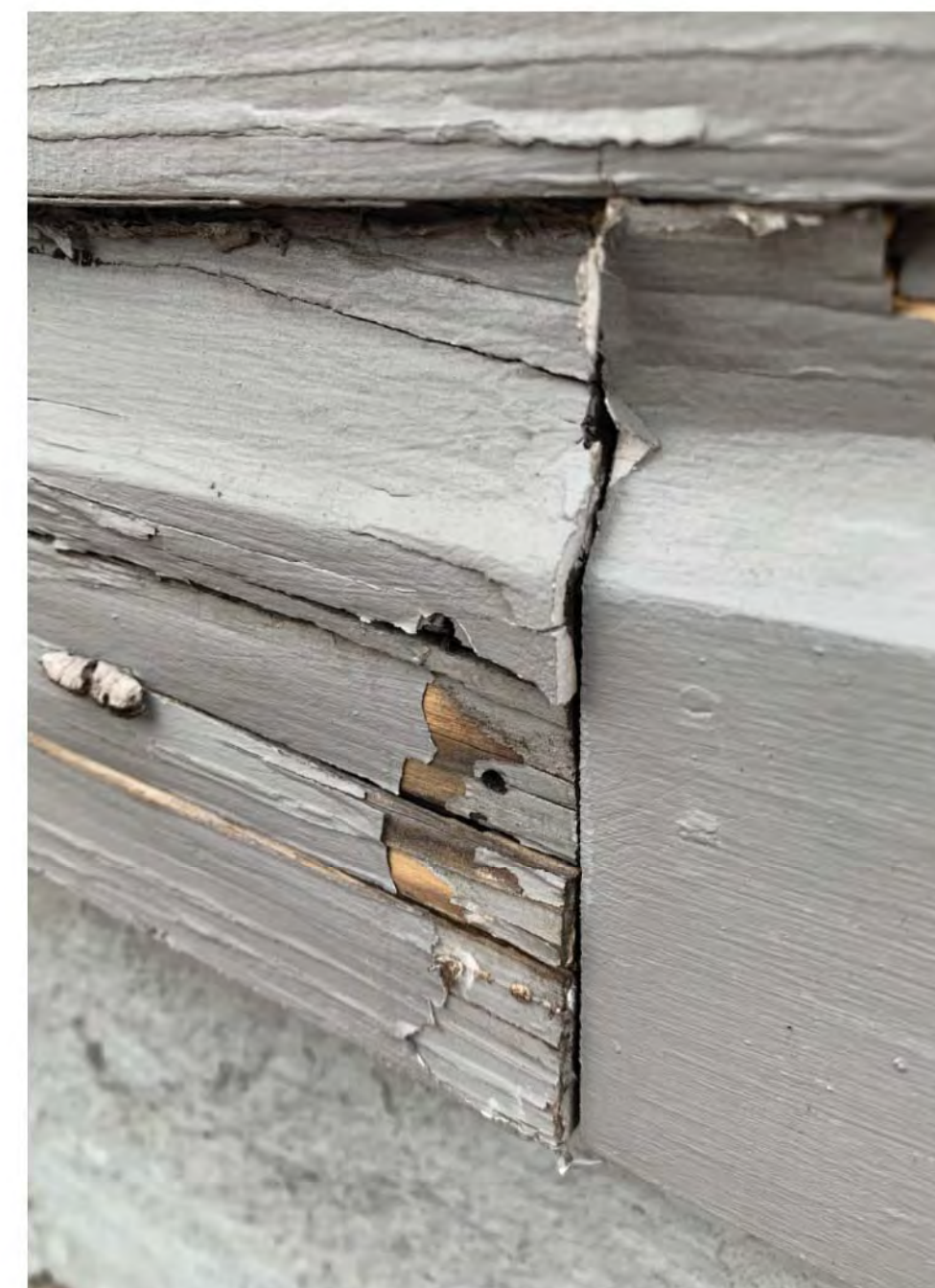
EXISTING PINE SIDING ROT AT NORTH WEST CORNER
