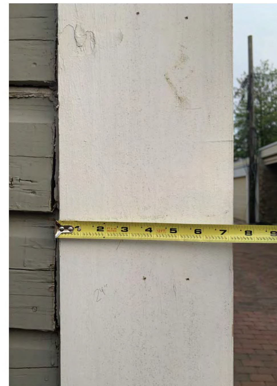
CORNER BOARD TO BE REPLACED (7-1/4") - NORTHWEST CORNER OF 3274 P ST. NW
