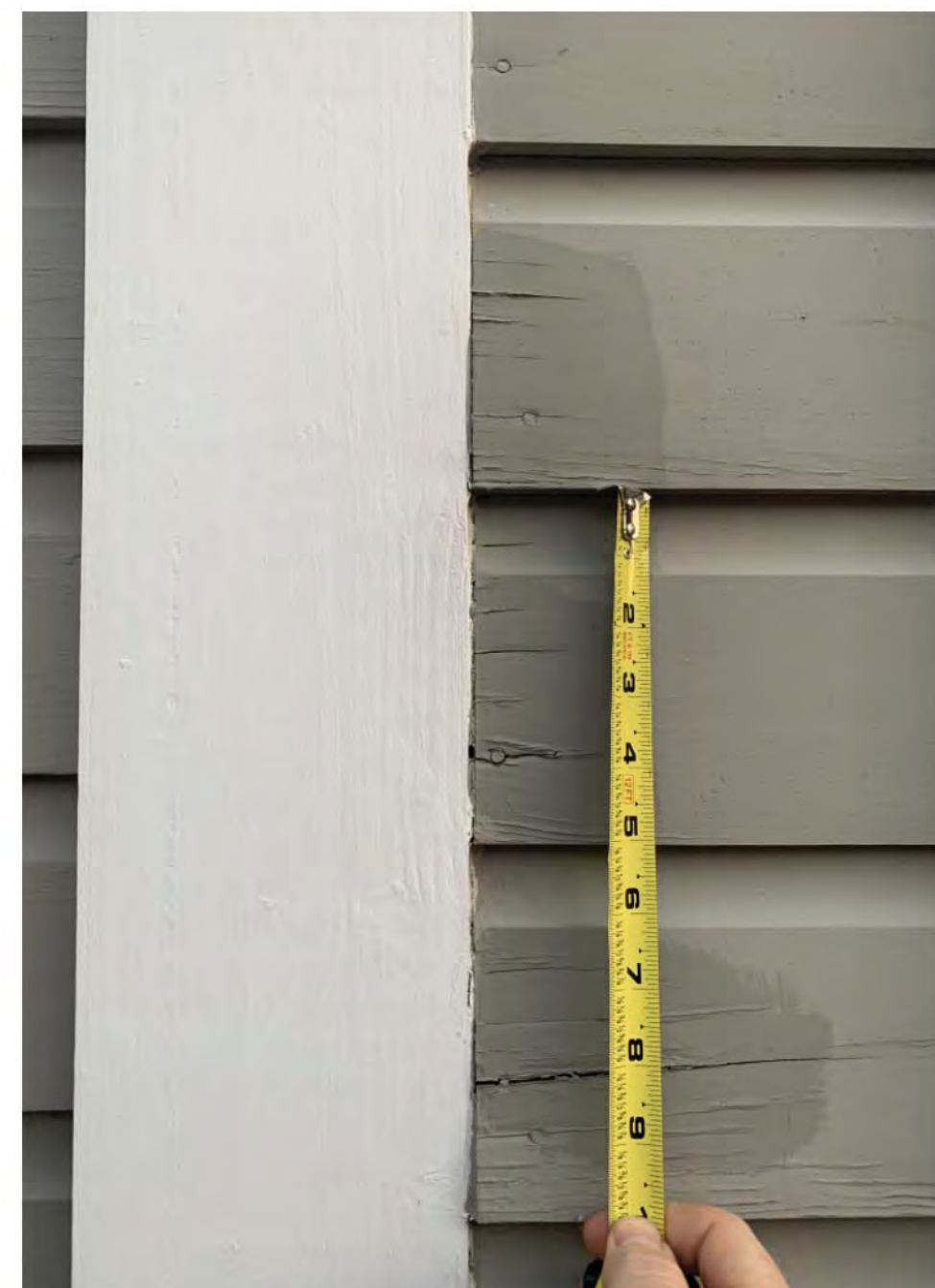
EXISTING SIDING EXPOSURE AT 3274 P ST. NW (PINELOCK SIDING TO BE REMOVED)
