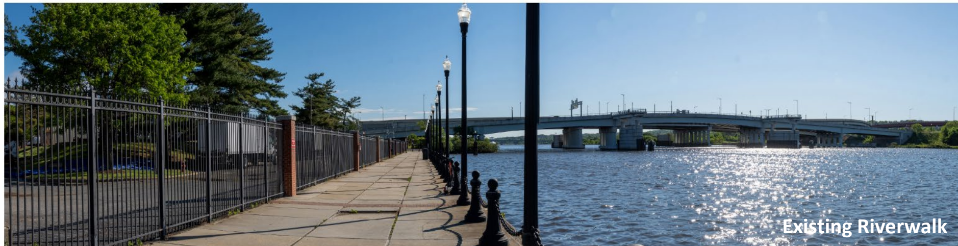
Condition of Existing Riverwalk Paving
