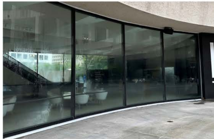
Thermal Envelope Deficiencies
