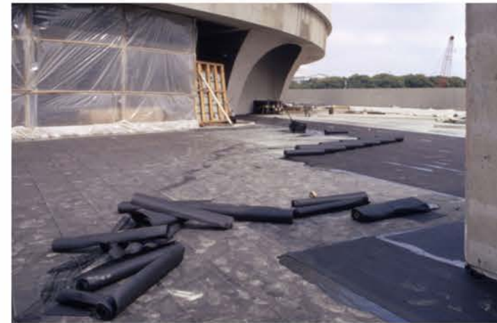
Waterproofing, Stormwater, and Flooding Deficiencies
