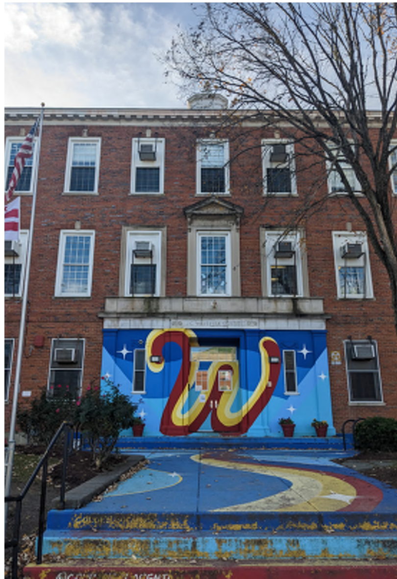
Paint TO BE REMOVED from Front Facade Cast Stone
