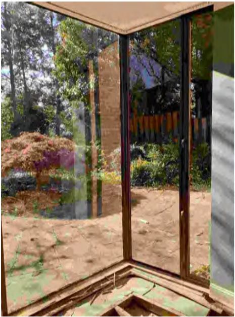
LEAK AT SILL
