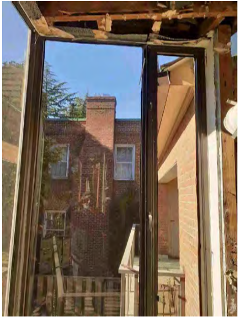
LEAKING AT HEADER
