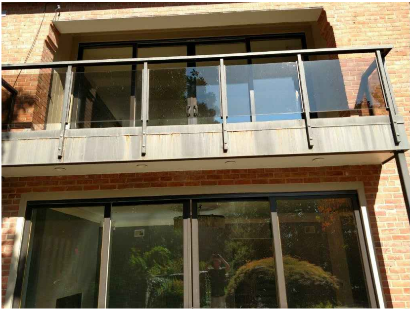
GAP AT HEADER
