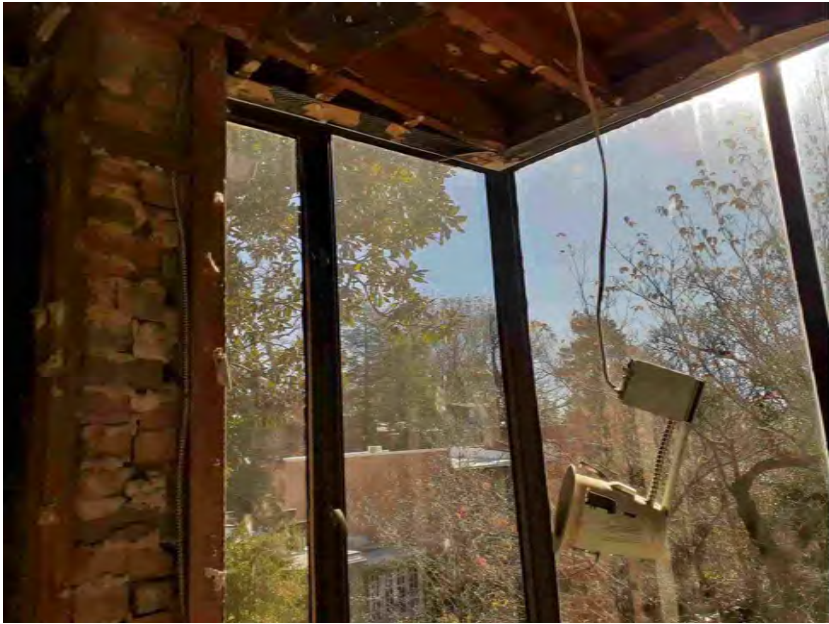
LEAKING AT HEADER
