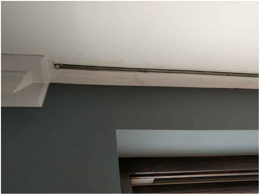
LEAKING AT CEILING
