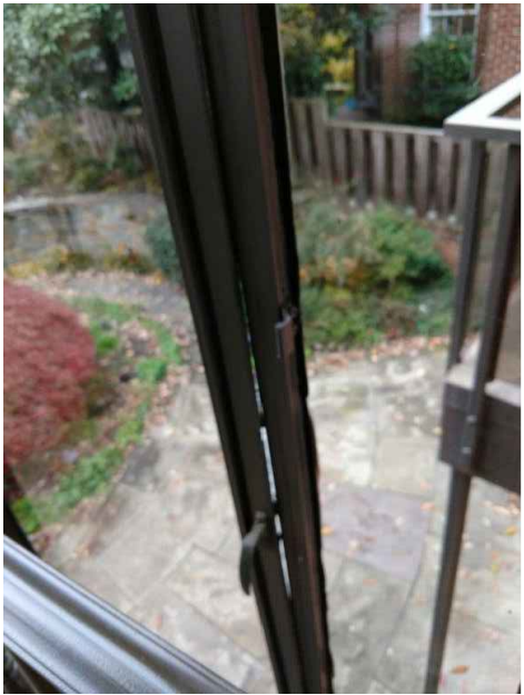
GAP AT LOCK
