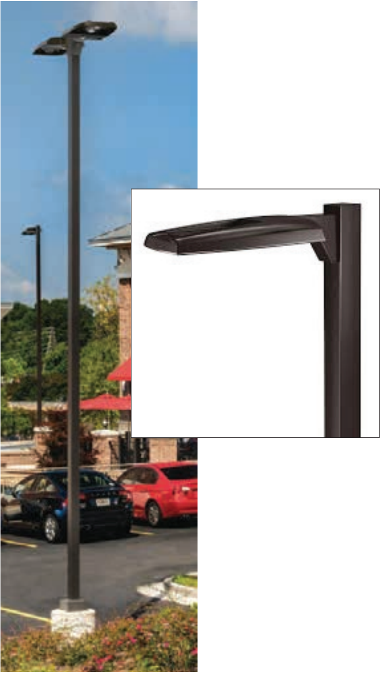
Lugman PRV double-arm pole-mounted light: Limited number of fixtures in the center of the Garage's top deck.
