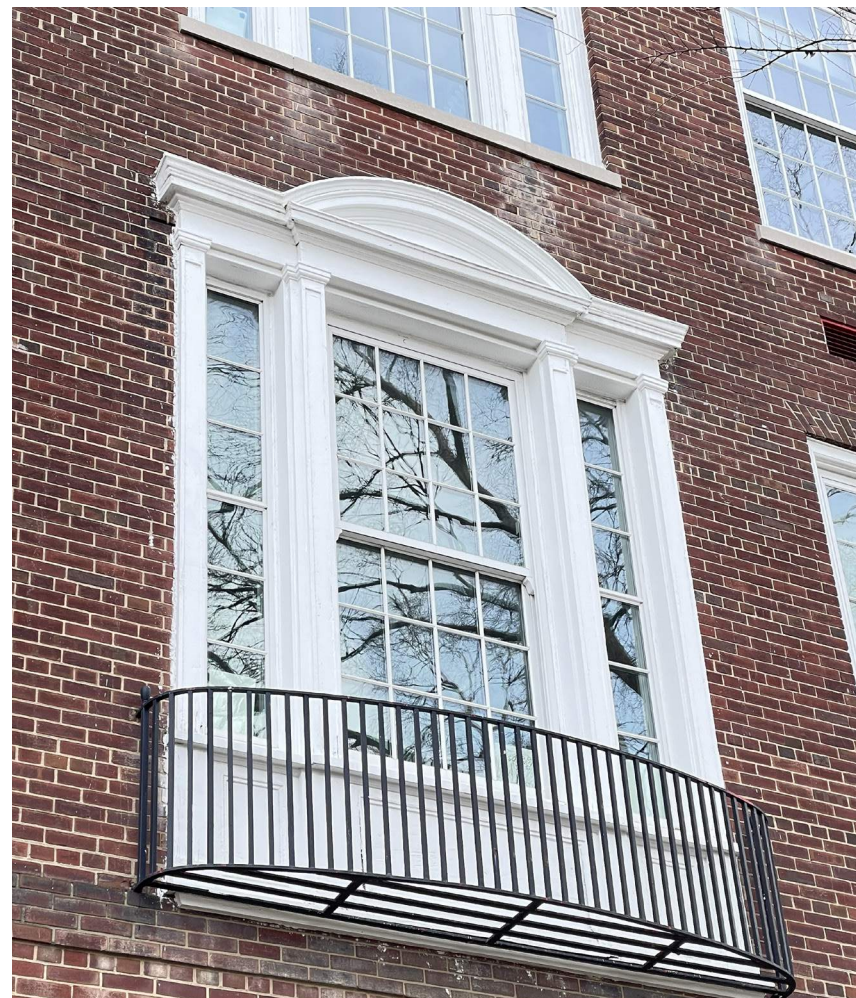
Window Detail at End Bay. Clean and repoint brick. Repair and repaint woodwork. Repair and repaint railing. Window to remain.
