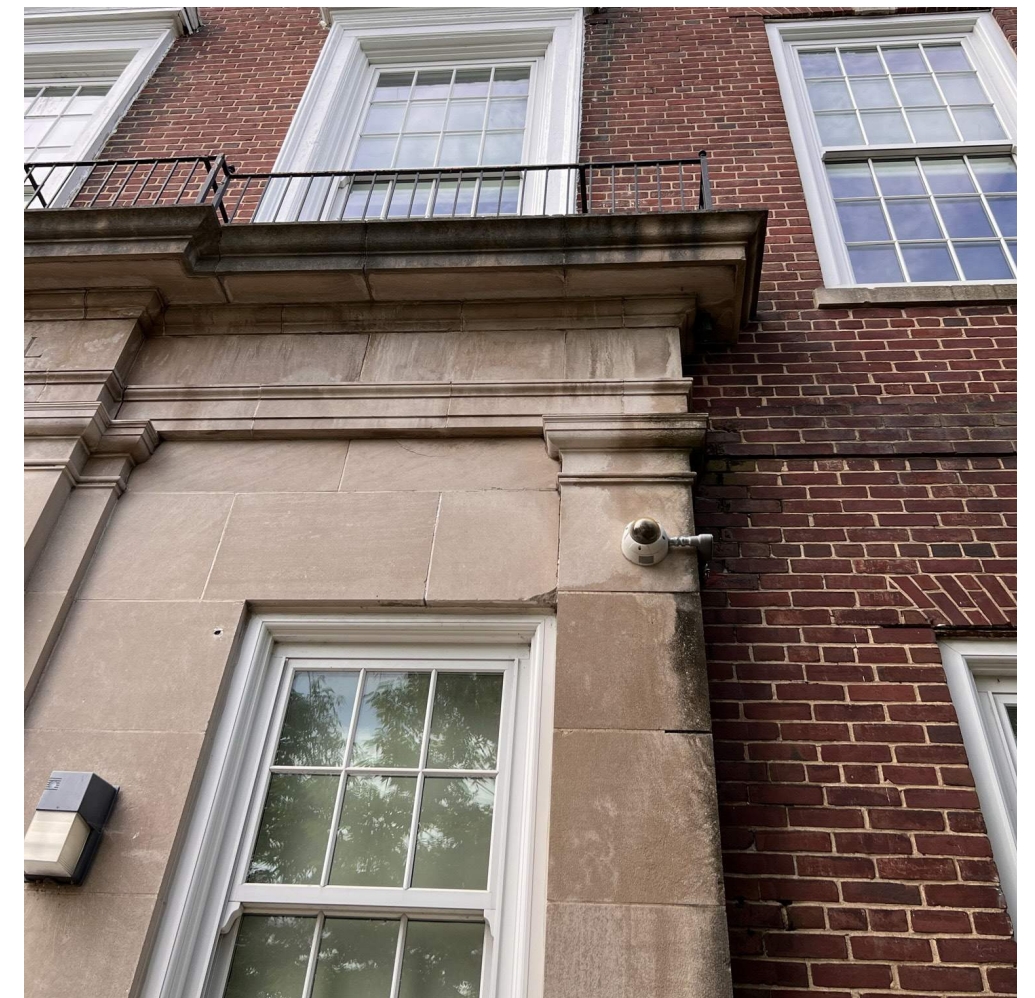
Historic Entry. Remove equipment, patch, install historically appropriate downspout, clean and repoint masonry, windows to remain.
