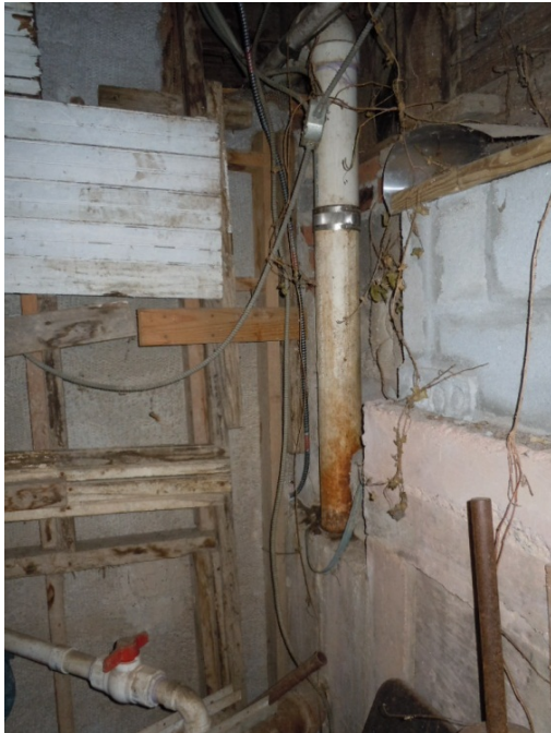
View of north west corner of east addition area showing CIP at base of wall.
