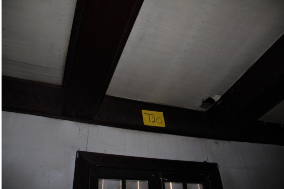
Task 20. Outcome: ceiling removal above W240 to expose concealed structure – no hidden structure in Board Room Ceiling, boxed beams are decorative (no concealed structure).
