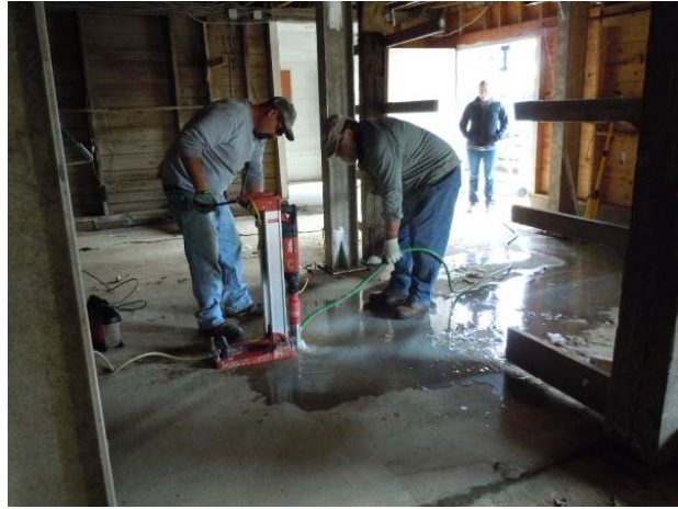
HPTC crew conducted numerous concrete core drilling to answer questions put forth by the structural engineer. (11/05/13, HPTC)
