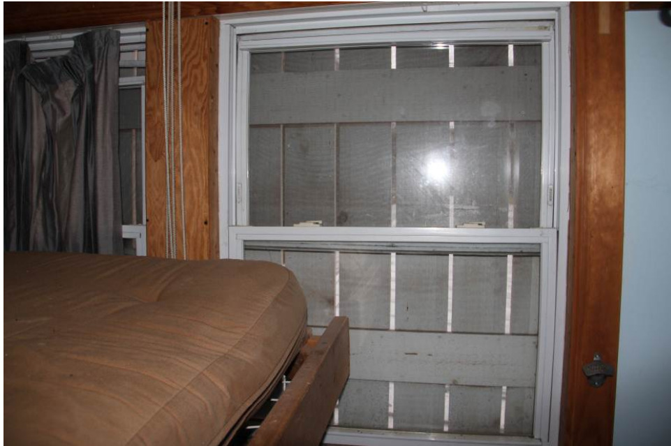
Interior view of a modern double-hung window (W317) in the North Tower (Room 304).
