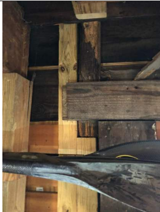
Photo #4: Replacement of historic wall studs of the south wall at 1 st floor level
