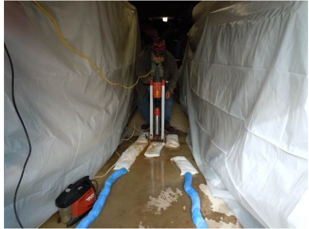
Preparations were made in the East Boat Storage Area to protect canoe club members' property prior to initiating a concrete slab core drill in this area as directed by the structural engineer. (11/05/13, HPTC)
