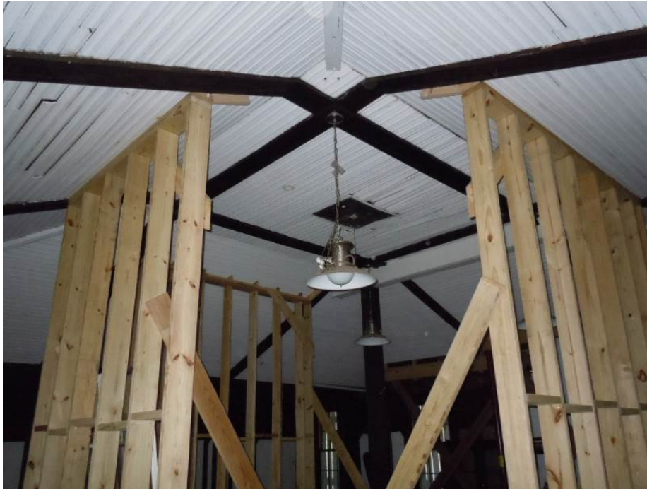
The Ballroom (Room 201) has painted beaded board paneling on the ceiling. Note loose and separating elements.
