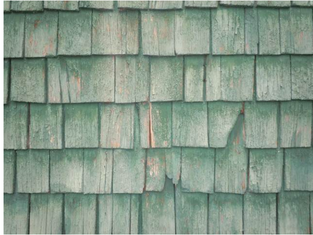
Typical painted wood shingle siding with approximately 5 inch exposure and random widths from 6 to 8 inches. Shingles are installed with random vertical staggered joints. (HPTC photo)
