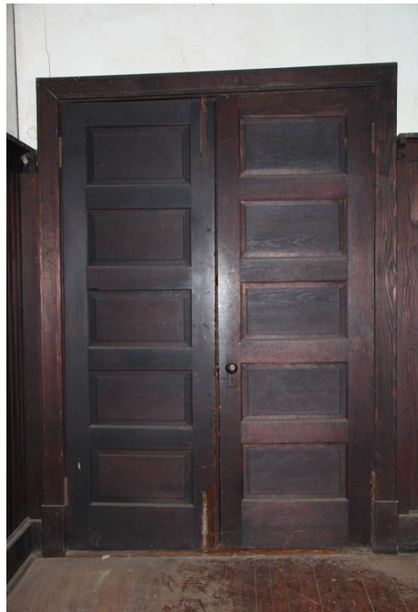
Five-panel doors to Board Room are from second phase of construction (ca. 1910). (HPTC photo)
