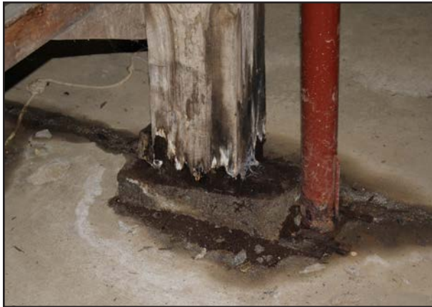
FIGURE 92 Rotted post on block in west boat storage area.
