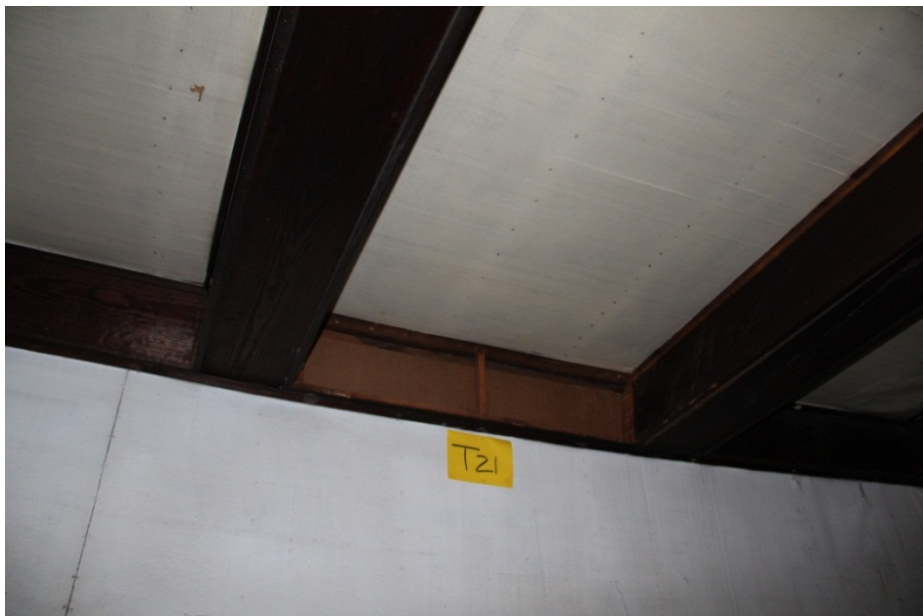
Task 21. Outcome: Interior north wall – ceiling finish removal to expose concealed structure. No hidden structure found, boxed beams are decorative (no hidden structure).
