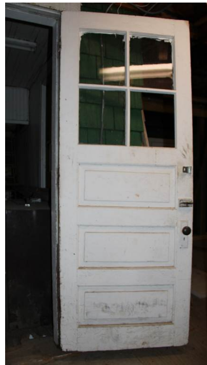
Opposite side of door (D206). This door is similar to door (D201).
