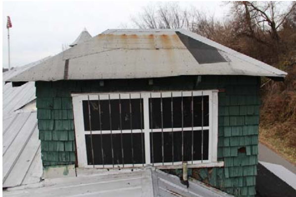
East elevation of North Tower hipped roof with non-standard installation of roof materials.
