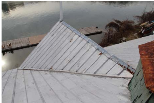
East roof slope of south cross gable with open valley and ridge cap. Note wooden mast at south end of ridge.
