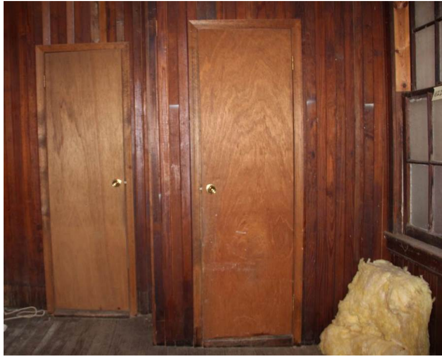
Doors (D211, D212) are modern luan doors installed in the Women's Toilet Room (Room 206).
