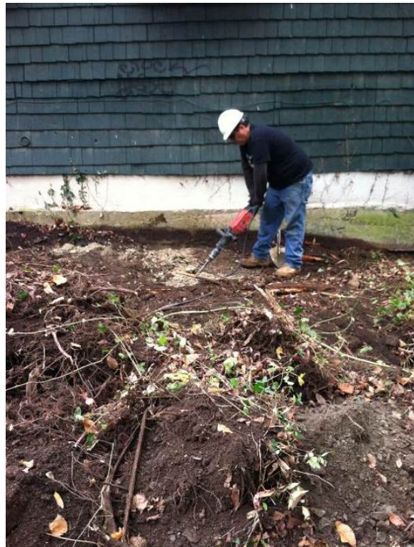
When machine excavation became problematic, hand excavation was attempted in order to uncover extent of concrete placements around base of building. (11/04/13, HPTC)
