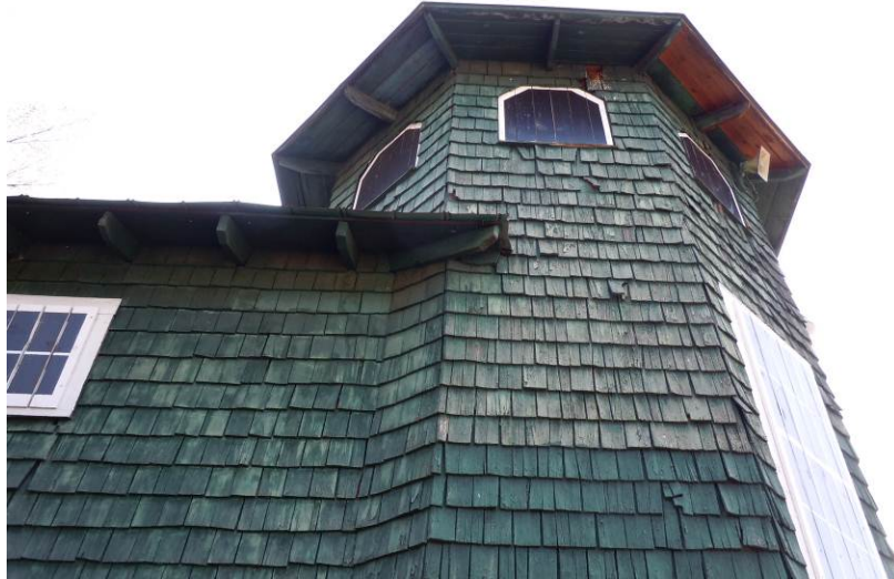
Roof sheathing and rafter tails are exposed on the roof overhangs. (HPTC photo)
