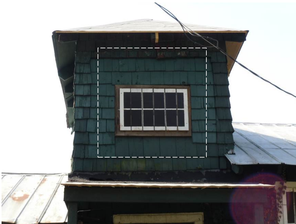
Exterior view of window (W319) on the north elevation of the North Tower (Room 304). This elevation may have originally had a door opening for access into the building from the former catwalk. Note the infilled area ( dashed line ) denoted by the contrasting shingles.
