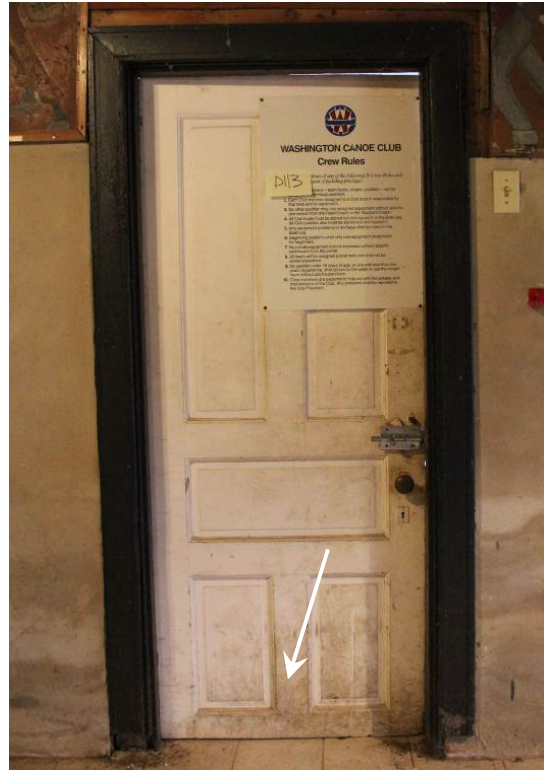
Door (D113) is similar to doors (D109, CL03A, and CL03B). The bottom rail (arrow) has also been trimmed.
