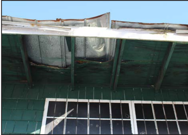
FIGURE 62 Detail of exposed sheathing and missing wood.
