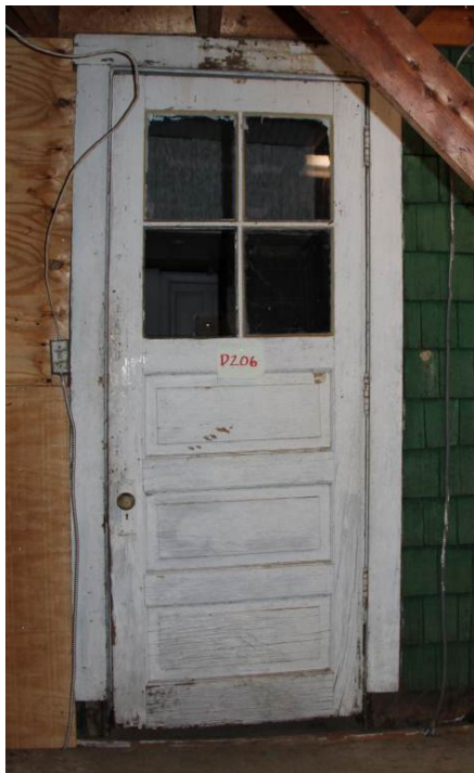
Original panel door (D206) leading from the North Entry Hall (Room 209) into the Workshop (Room 211).
