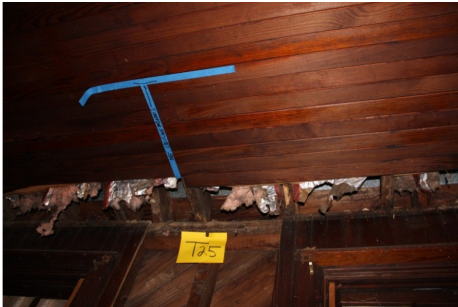
Task 25. Outcome: Interior wall sheathing removed to expose wall structure including base and top plate of wall and connection with ceiling joists and roof rafters.
