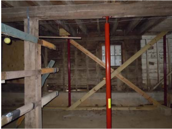
Temporary pipe columns (red) and wood cross-bracing was added by the NPS CHOH Maintenance Team according to stabilization plans by a structural engineer to correct deficiencies in the buildings superstructure. (10/23/13, HPTC)
