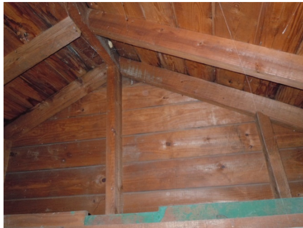
View of underside of simple gable truss roof frame at the Women’s Locker Room. The locker room was constructed in two phases and minor variations occur between the two sections of roof frame.
