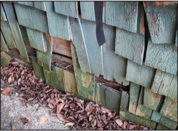
FIGURE 52 Detailing of weathered, cracked, missing, and dislodged shingles on the west elevation.
