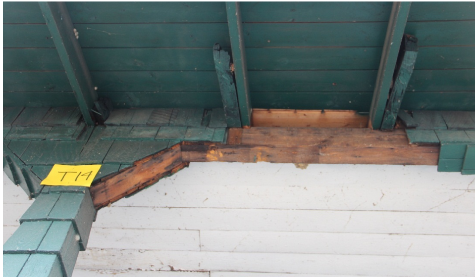
Task 14 Outcome: structural post, bolster (or half diamond capital) and porch breast beam structure revealed under original shingle cladding. Note solid beam used to support roof frame in this area of Phase 1 construction. See task 18 for comparison where a double beam was used in lieu of a solid hewn beam, as above.
