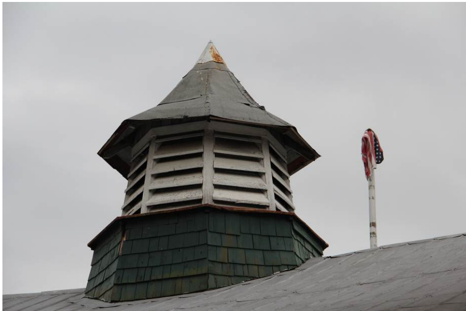
The shingle siding on the base of the cupola matches the siding on the perimeter of the building.
