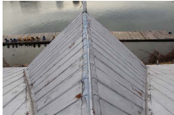
Ridge line of gable with mast at south end showing open valley flashing at either side.
