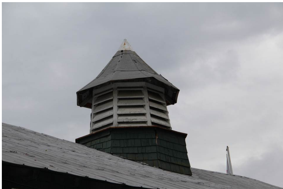
The louvered octagonal cupola with conical roof (covered with mineral surfaced roll roofing and original pinnacle cap painted white) serves as a ventilator for the Ballroom below. (HPTC photo)
