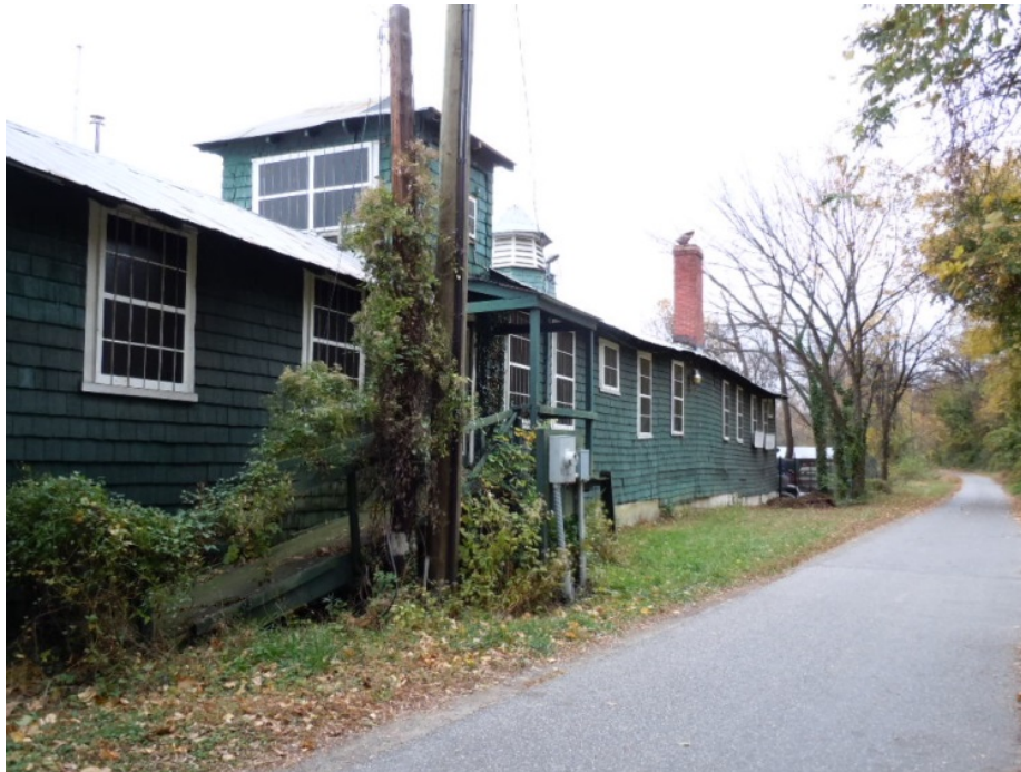
A wood ramp is installed over the stairs (ST03) leading to the north entrance door (D208) on the north elevation.
