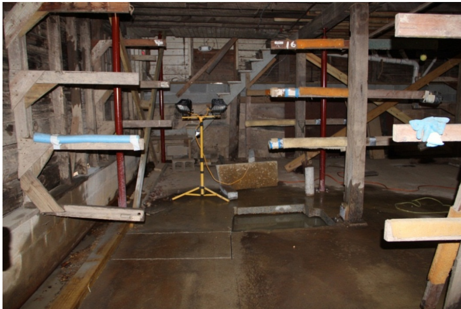
Task 12: Overview of Slab Saw Cut areas 1 (at post) and 2 (at exterior wall).
