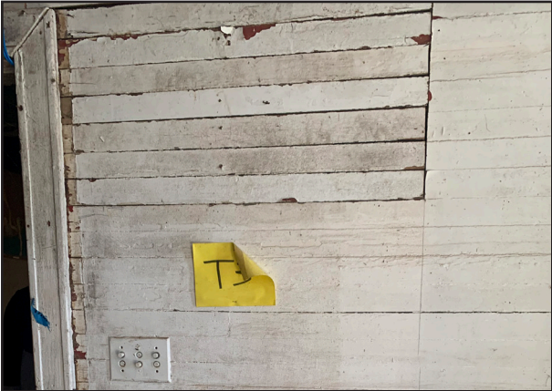
FIGURE 119 Wood in hallway on first floor is of early 20th C. wood construction. The wall cavity was filled with silt from periodic inundation during Potomac River floods. Portions of the wall were removed in 2014 for investigation.
