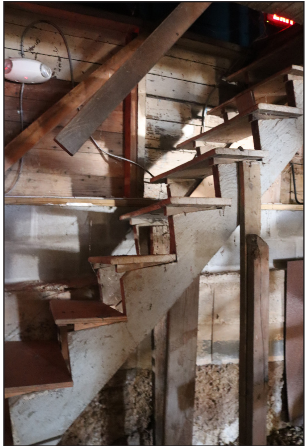
FIGURE 112 Non-compliant and flimsy stairs in northwest corner of West Boat Storage Area.
