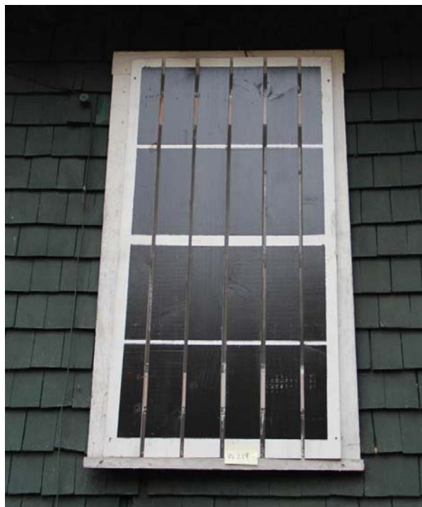
Typical painted wood cover on the exterior side of the double-hung windows on the north elevation.
