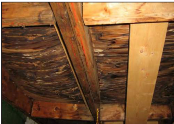
FIGURE 94 Severe rot in roof sheathing over workshop.
