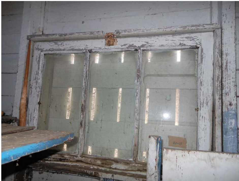
Typical 3-lite hopper window located above the lockers in the west wall of the Men's Locker Room (Room 203).
