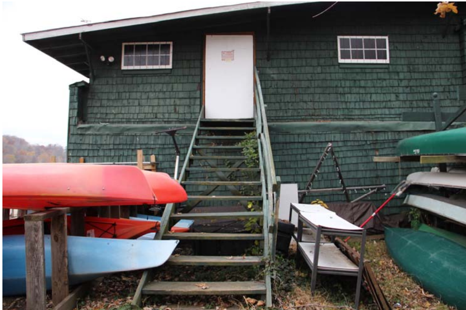
The stairs at the east entrance to the building are unstable and non-compliant with building codes.
