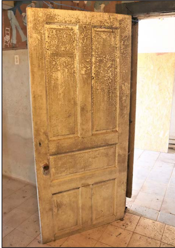
FIGURE 121 Original five-panel wood door with original hardware. Note that the door was cut down to fit in the opening after the floor was raised.
