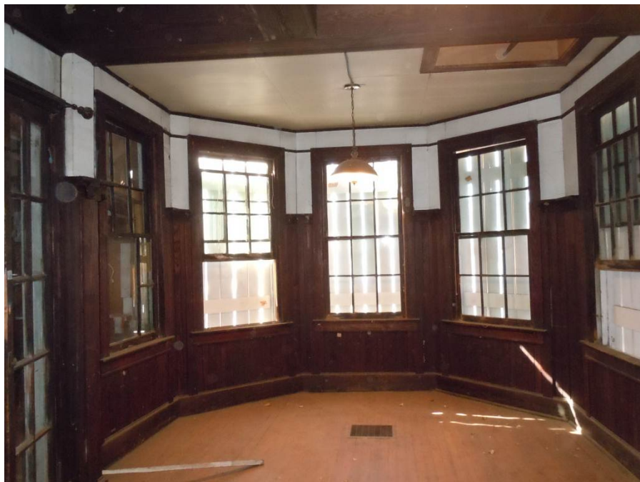
Double-hung windows (W236-W239, W248) located in the tower portion of the Board Room (Room 208).
