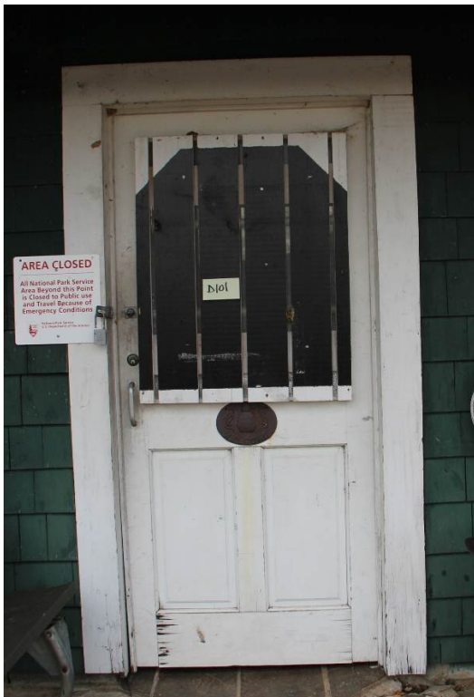
Exterior view of glazed door (D101) on the south elevation. Painted wood planks are installed over the glass panes.
