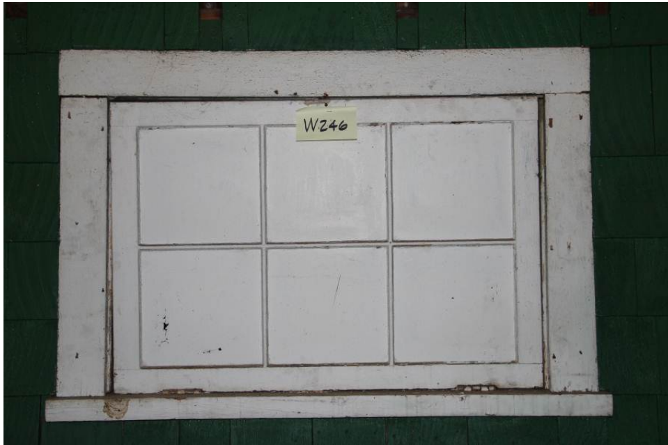
Typical hopper window in the south wall of the Women’s Locker Room (Room 210).
