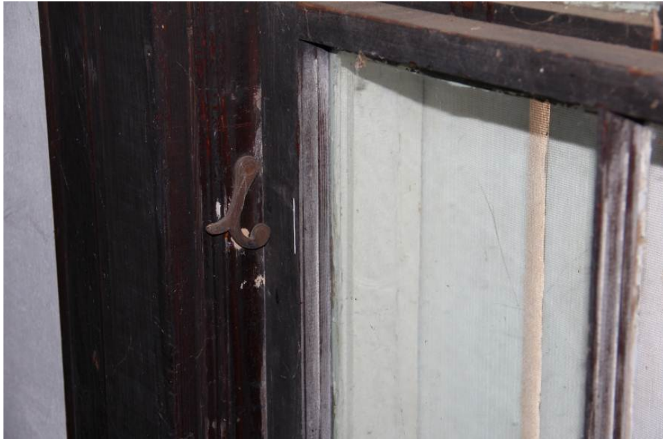
Detail of a sash holder on double-hung windows in the Ballroom (Room 201).
