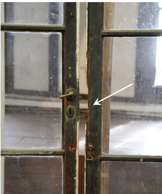
Detail of interior hardware on double casement windows. Note wood damage on stile (arrow).
