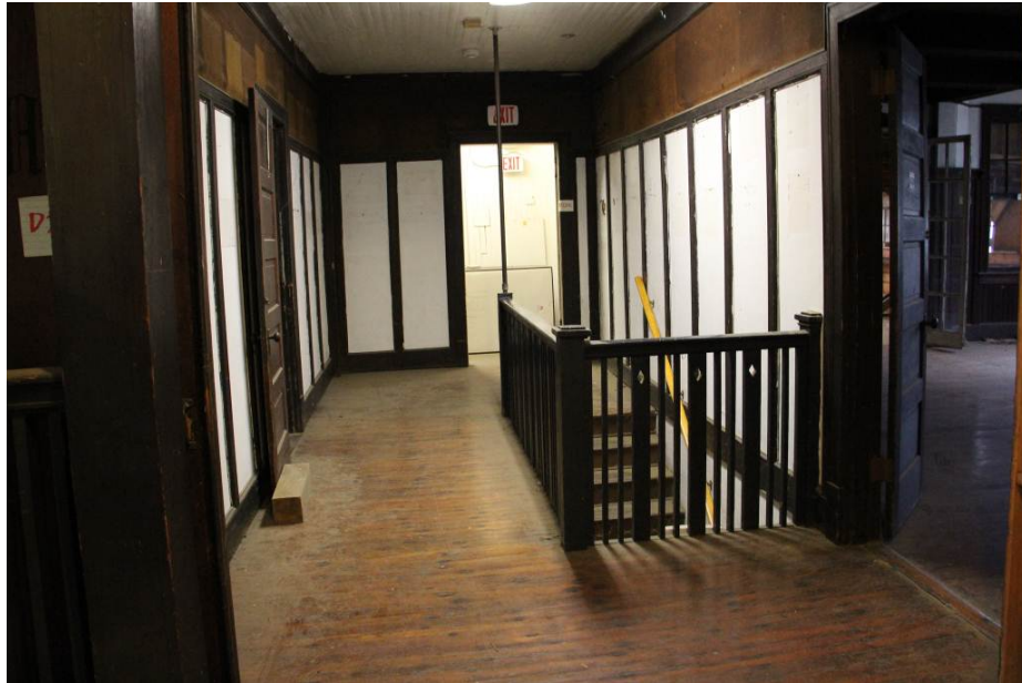
Vertical wall panels with white-painted fabric over dark stained beaded board paneling, wood strip beaded ceiling, wood plank floor, stair balustrade and newel posts are all character-defining features in the Entry Hall (Room 207) on the second floor. (HPTC photo)
