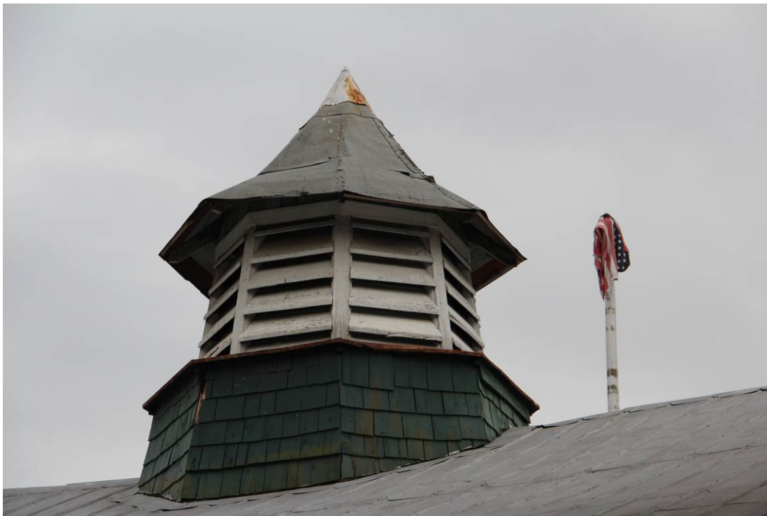
Louvered cupola with conical roof on the ridge of the main roof. (HPTC photo)
