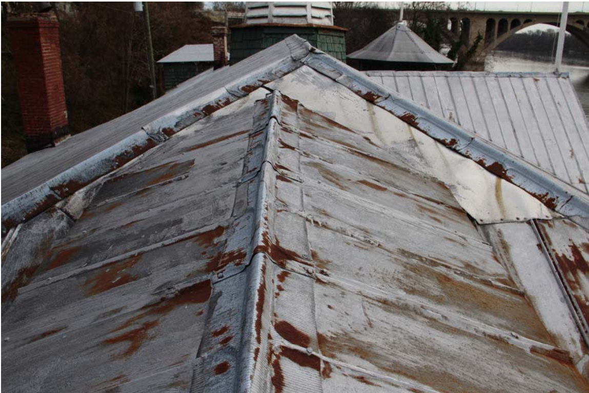
Deteriorating existing metal roof finishes and flashings.
