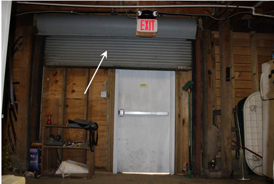
Interior view of door (D114) showing the door infill and man-door. The overhead roll-up door is still installed (arrow).
