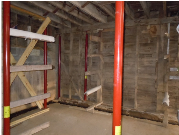
View of interior NW corner of building at ground level with drainage troughs cut into floor slab against north (rear) wall and west (left) wall of building (11/05/13, HPTC).
