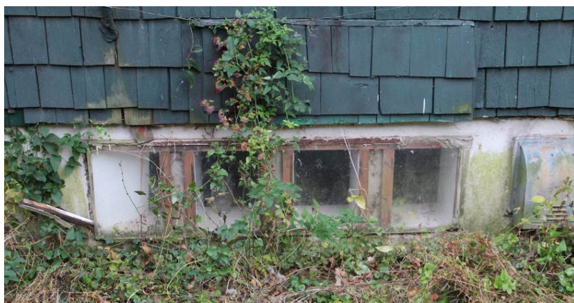
Exterior view of the window opening on the first floor on the north elevation. The exterior of the opening is covered with an acrylic panel.
