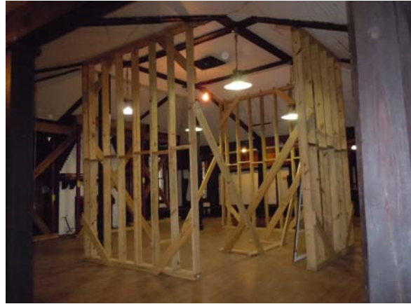
Cross-bracing was added in the Ballroom on the second level to assist in the support of the deflecting light-weight wood roof frame. (10/23/13, HPTC)
