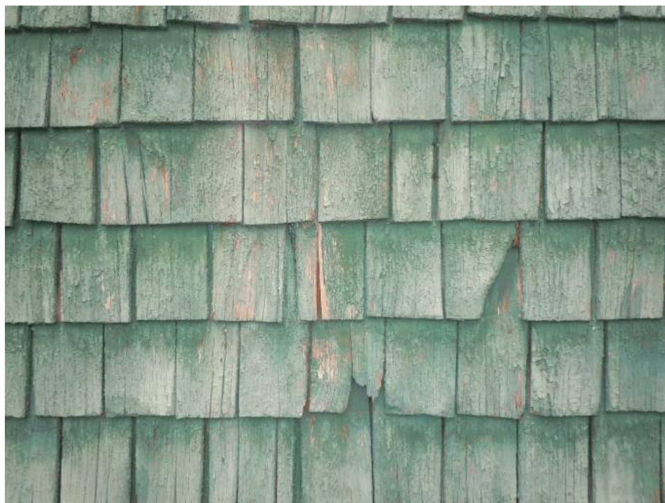
Detail of shingle siding with cracked and broken shingles and failing paint finish.
