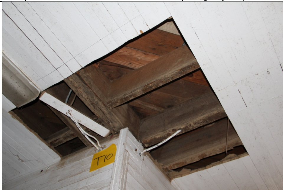
Task 10 Outcome: Floor frame structure revealed. Diagonally installed sub floor visible fastened to floor joists. Spacing, configuration, condition and perforation of frame revealed.
