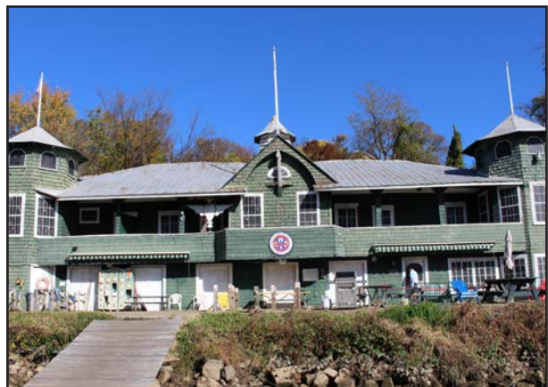
FIGURE 66 Roof on south elevation, looking north floating dock. Extensive rusting visible.
