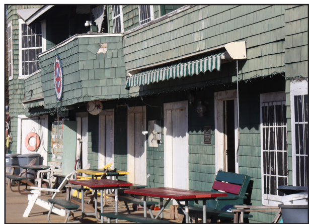
FIGURE 58 Balcony without brackets. Noticeable sag in the cantilevered balcony structure visible.
