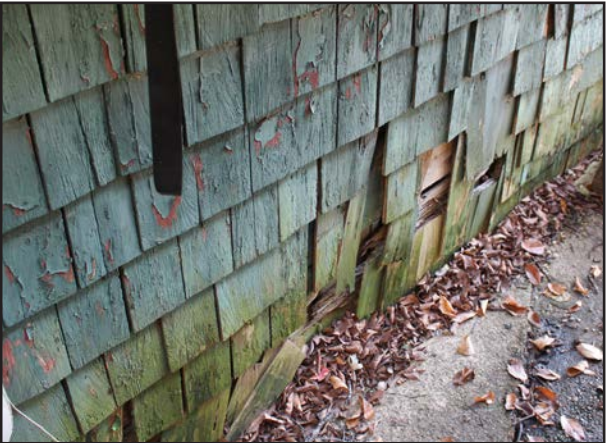
FIGURE 51 Detailing of weathered, cracked, missing, and dislodged shingles on the west elevation. Mold visible. Red paint (possibly original) exposed.
