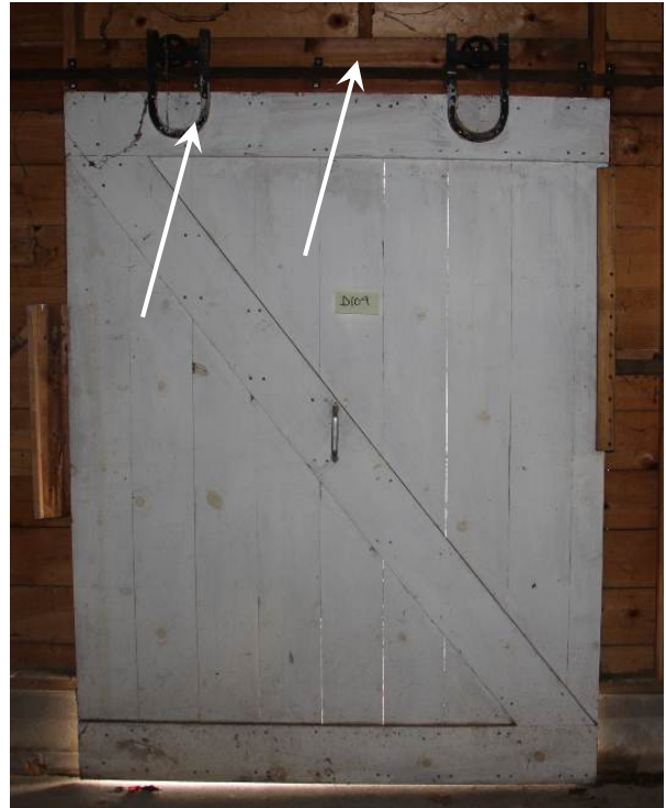
Interior view of door (D104). Note the barn door rollers and track (arrows) at the top of the door.
