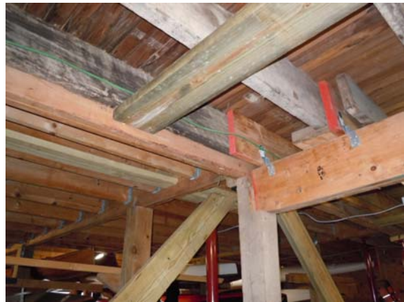
Detailed supplemental framing and additional supports stabilized the East Boat Storage Area allowing access by the WCC membership. (11/12/13, HPTC)
