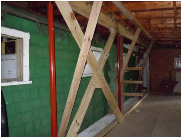
Shear bracing added on the second level along the south wall of the Women's Locker Room adds to the stability of the under-structured addition. (10/23/13, HPTC)
