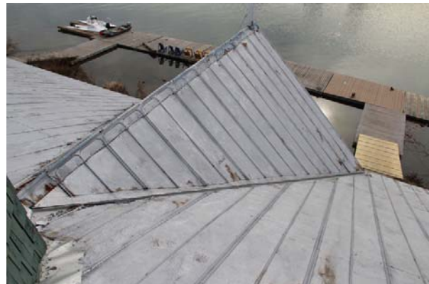
West roof slope of south cross gable with view of cupola base flashing to the north.
