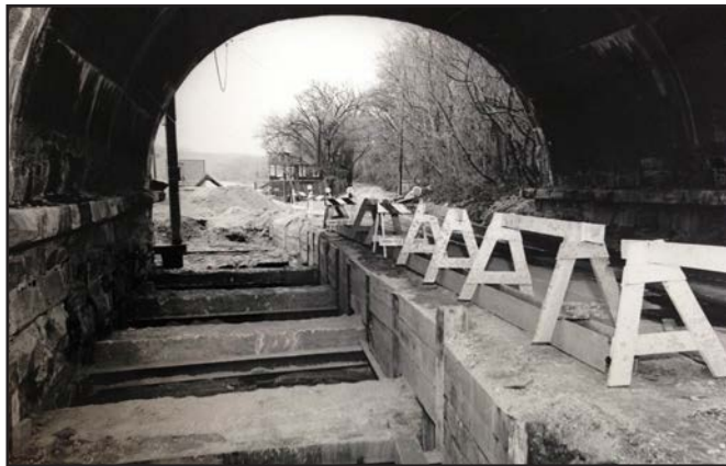
FIGURE 26 Installation of Potomac Inceptor Sewer Line, looking west, .c. 1965. Washington Canoe Club.
