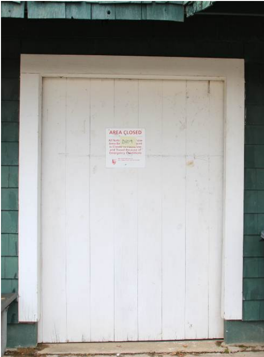
Exterior view of a typical sliding door (D104) in the West Boat Storage Area (Room 101).
