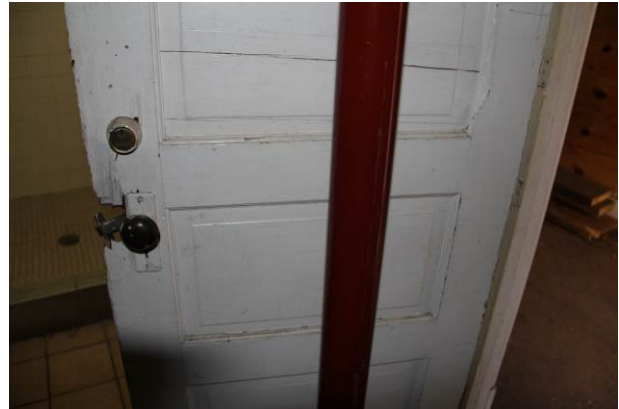
The panels of door (D210) are cracked and the door is broken at the latch.
