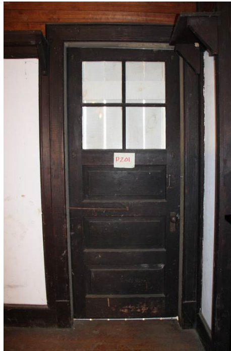
Original 3-panel, 4-light wood door (D201) leading from the Ballroom (Room 201) to the Balcony (Room 212).
