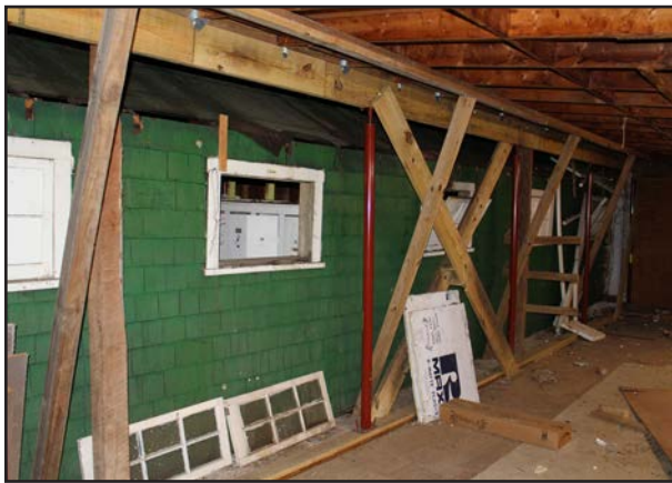
FIGURE 75 Window openings on south side of Ladies Locker Room (originally exterior wall). Some windows have been painted over while other windows have been removed from their frames.
