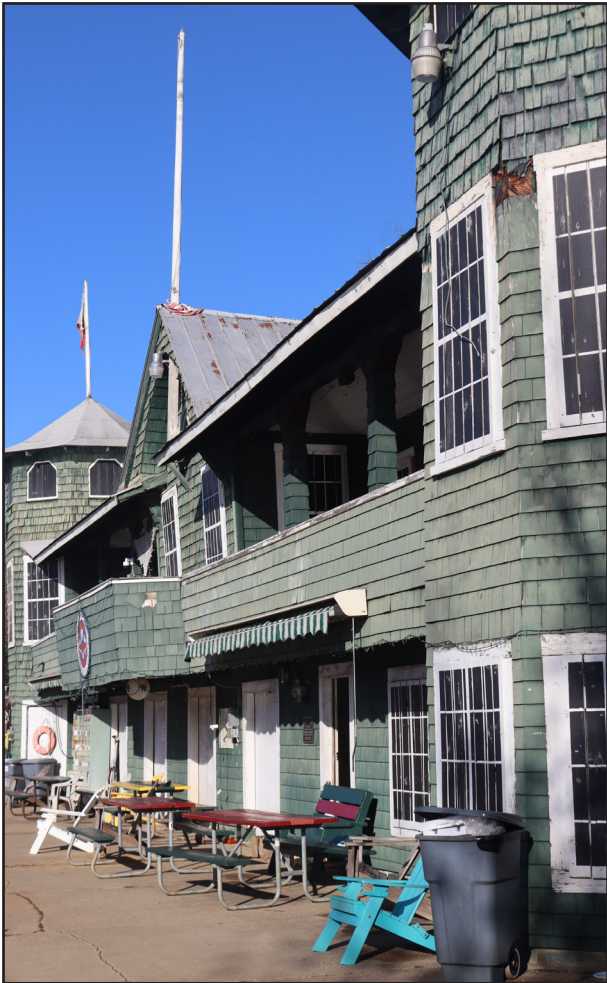
FIGURE 48 Green painted wood shingle siding with white trim on south elevation. Areas of replacement and missing shingle evident. Note that the balcony structure is leaning away from the building.
