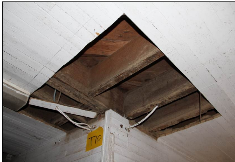
Example of historic fabric removal by HPTC to expose the historic wood frame of building for assessment by structural engineer consultant. [HPTC]
