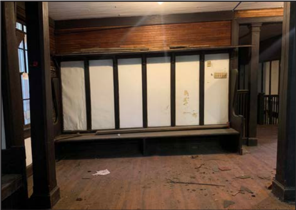
FIGURE 117 Wall treatment in Ballroom. Note areas of peeling and bubbling paint.
