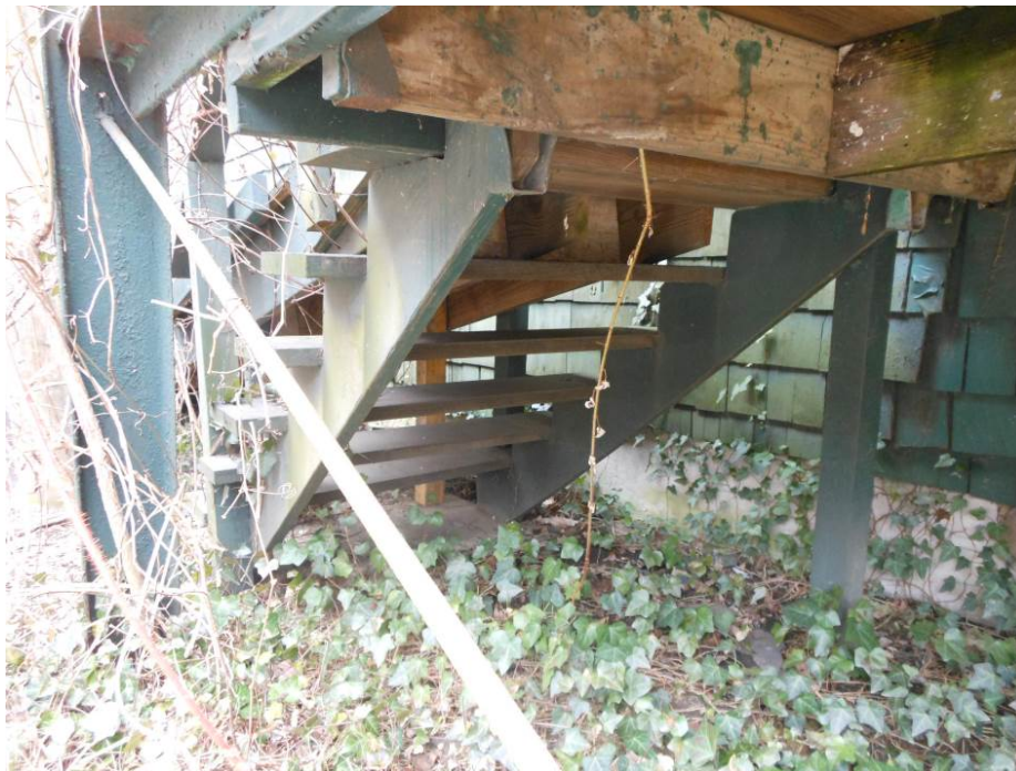
The wood stairs (ST03) are still located under the wood ramp at the north entrance.
