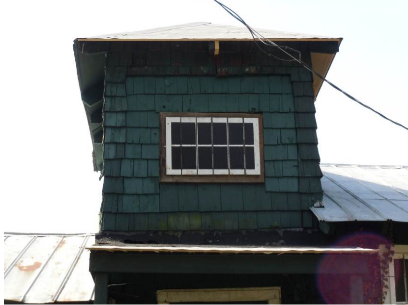
Hipped roof over the North Entry Tower on the north elevation. (HPTC photo)
