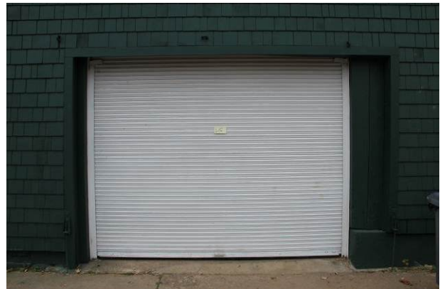
Exterior view of typical overhead rollup door on the south elevation of the east addition. (HPTC photo)
