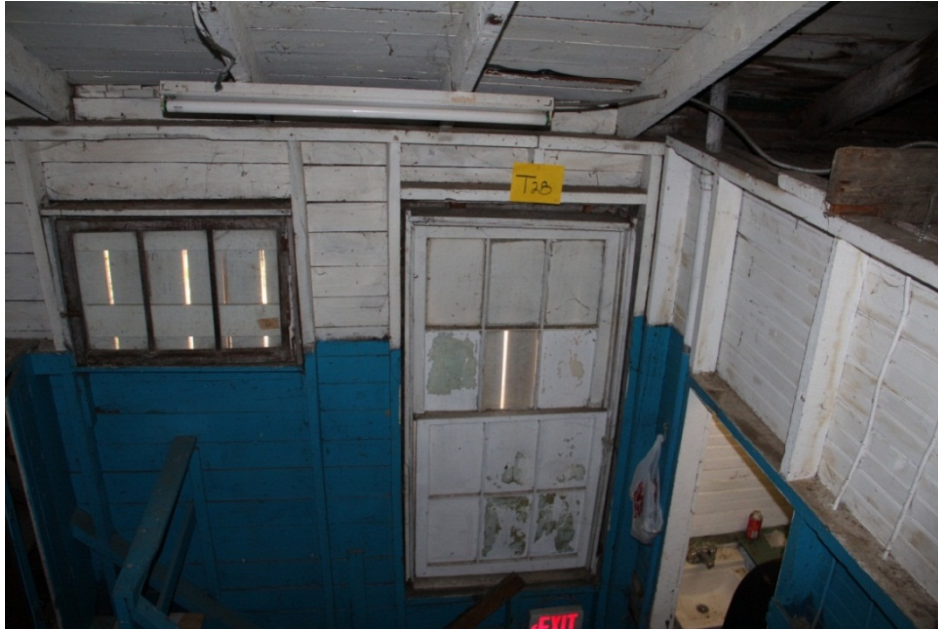
Task 28. Outcome: No fabric was removed as structural members are exposed above wall line in locker room and above the ceiling level of the Men’s Toilet room (photo right).
