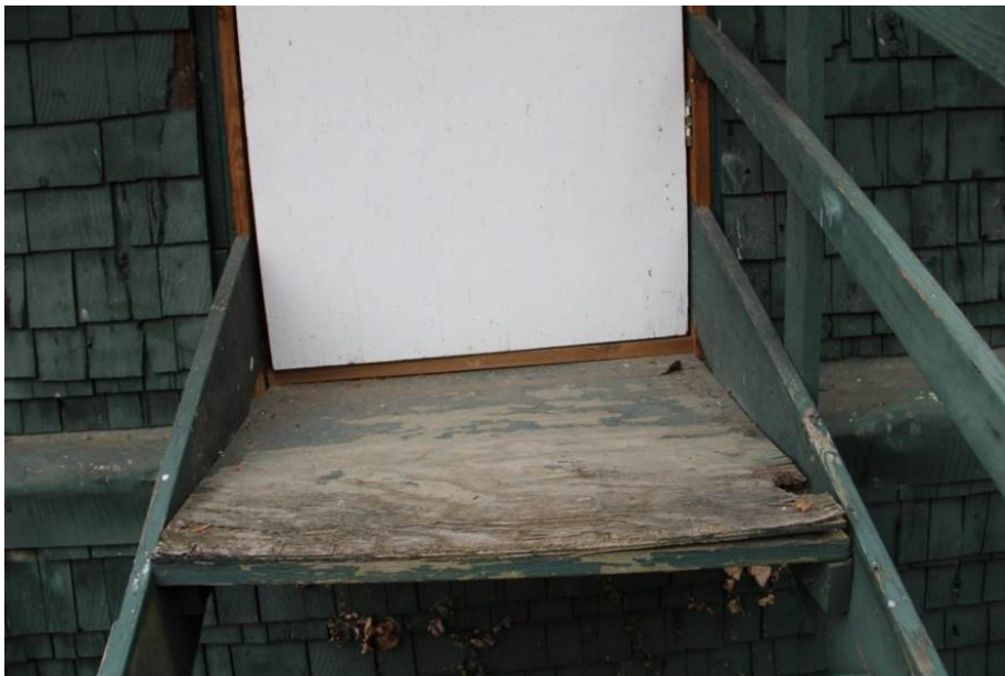
Deteriorated plywood landing at the top of the east entrance stairs (ST04).
