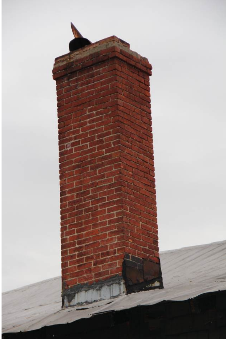
West brick chimney (CH01) with corbelled top courses. Brick is laid in common running bond. (HPTC photo)
