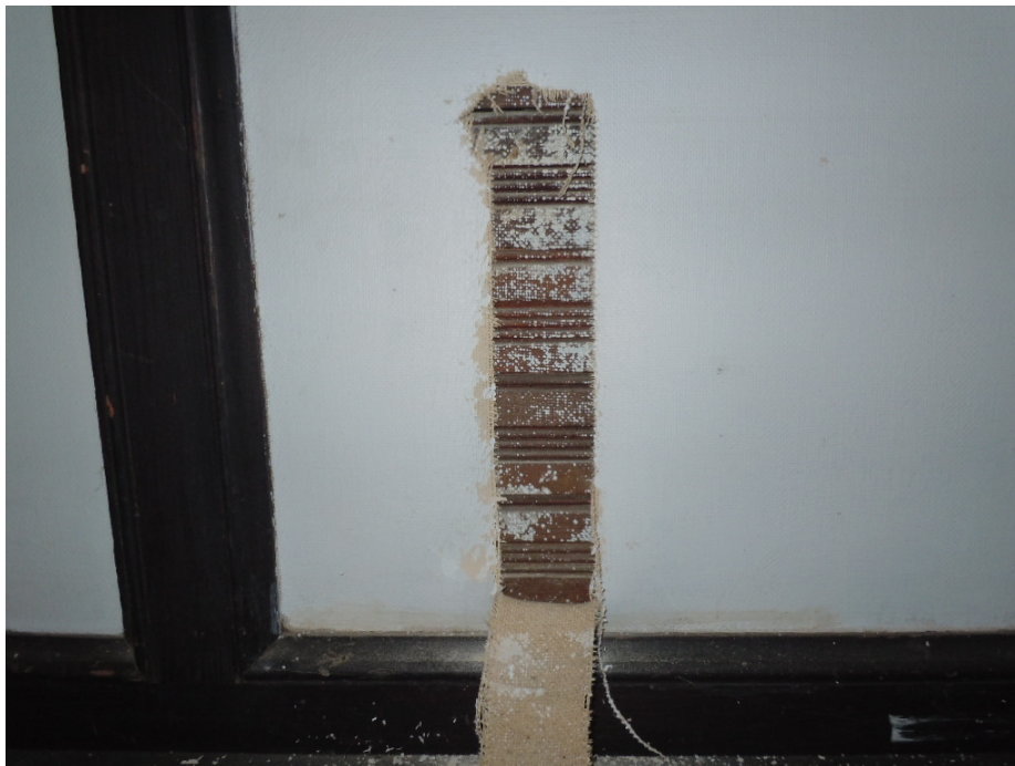
A piece of painted wall fabric is torn on a wall in the Ballroom (Room 201) which reveals the beaded board paneling underneath.
