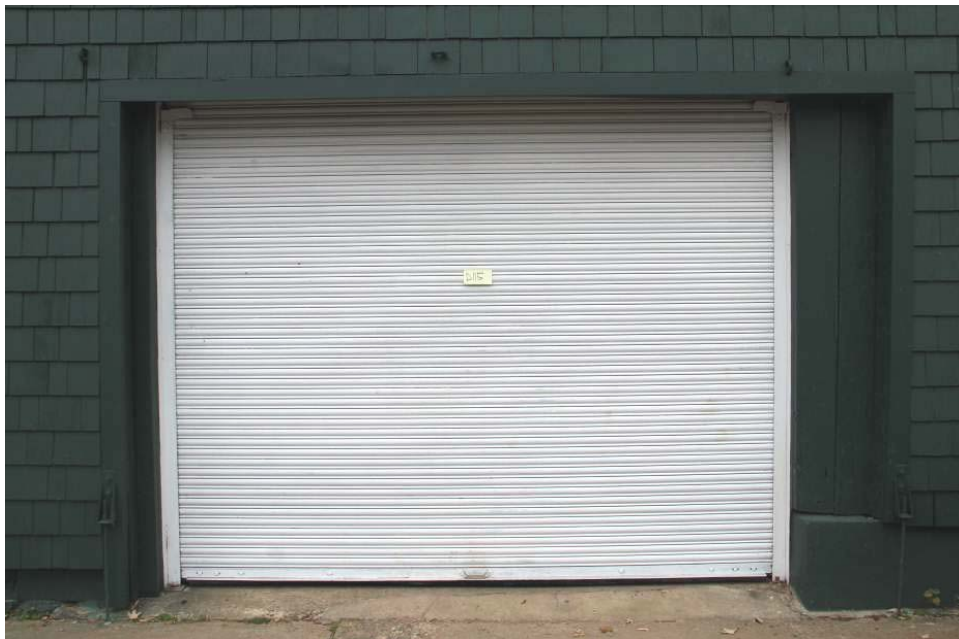
Exterior view of typical overhead metal roll-up door in the East Boat Storage Area (Room 106).
