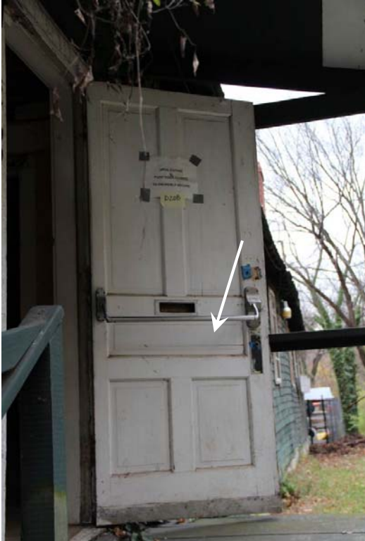
Interior view of Door (D208). The original door hardware has been removed and replaced with panic hardware (arrow).
