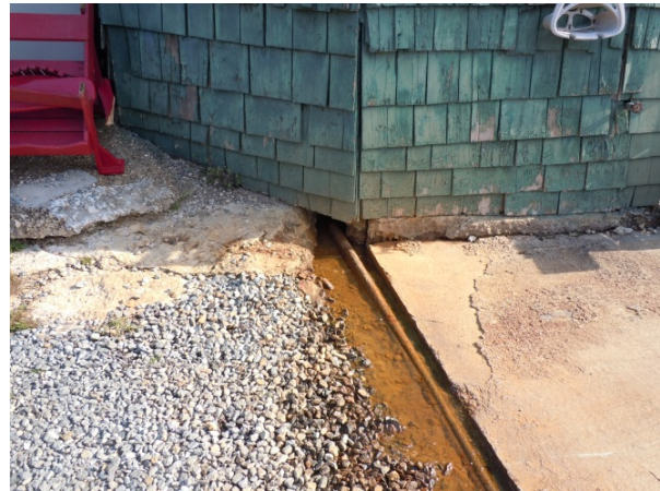
Detail at SW corner with drainage trough cut into concrete slab with water discharging from north elevation area (4/19/13 HPTC).
