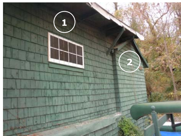
Detail of roof overhang on Workshop (1) and gable end of Women's Locker Room (2).
