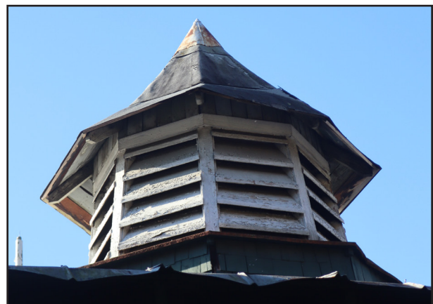
FIGURE 54 . Detail of deteriorated wood louver panels.
