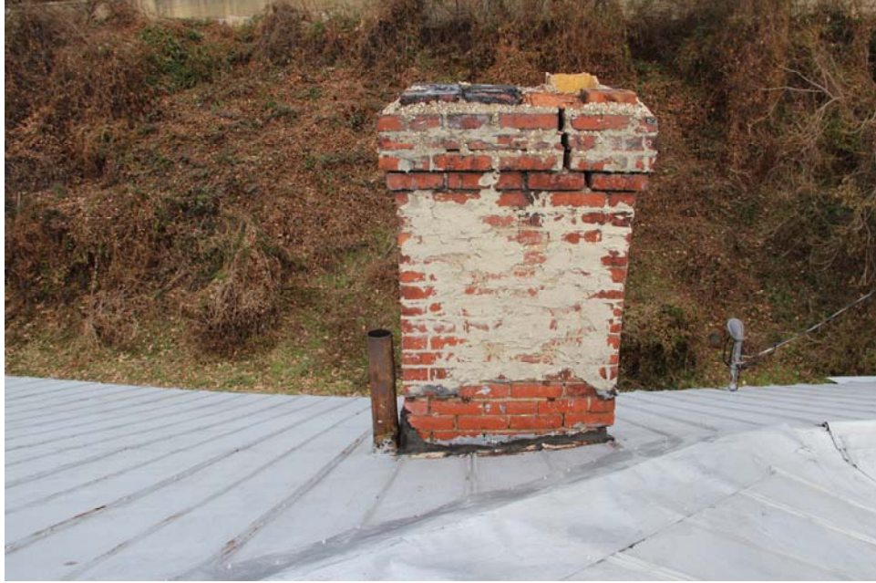
The brick chimneys are failing and lack adequate flashing.
