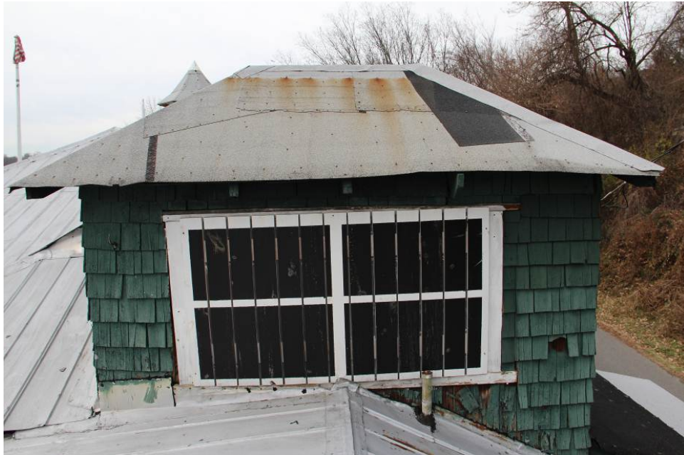
Exterior view of windows (W317, W318) on the east elevation of the North Tower (Room 304).
