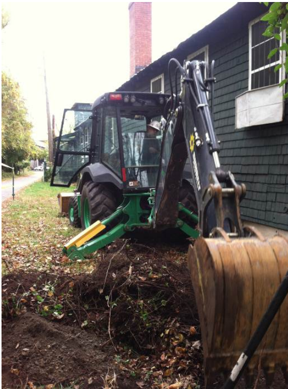
Exterior excavations conducted by the HPTC crew as part of the project of the north elevation attempted to determine the extant foundation conditions. (11/04/13, HPTC)
