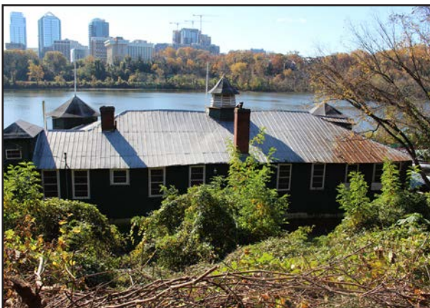
FIGURE 65 Roof on north elevation, looking south from C&O Canal toepath. Extensive rusting visible at northwest corner of the building.
