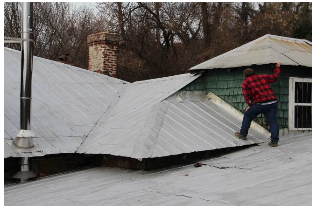
Roof observation and assessment was conducted in late December on an above average temperature day. (12/20/13, HPTC)
