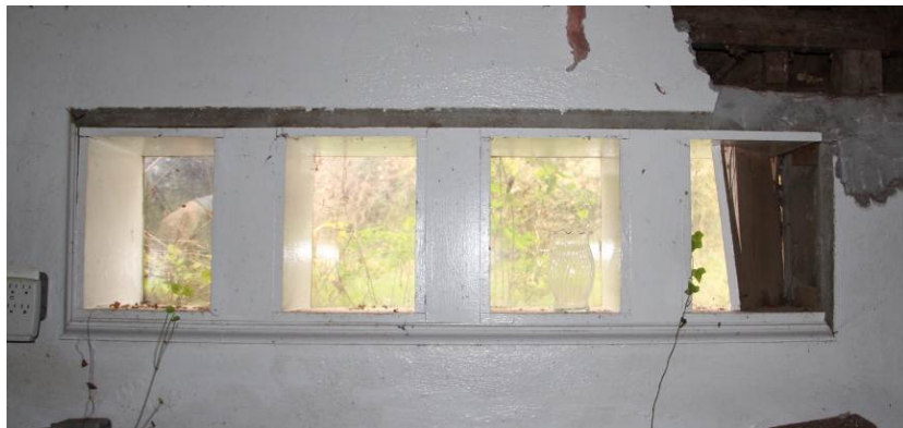
Interior view of the window opening (W110) in the north wall of the Kitchen (Room 103) on the first floor.
