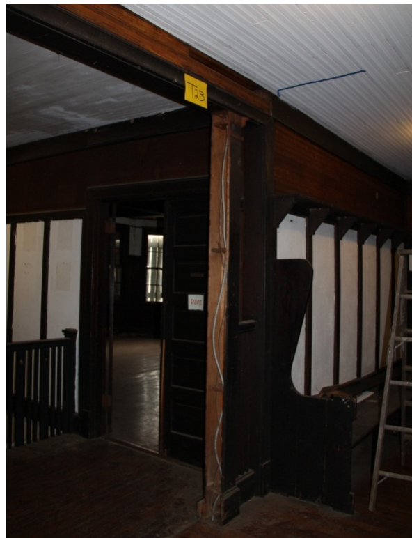
Task 23 Outcome: revealed architectural treatment at opening is decorative – no concealed structure in ceiling or at boxed columns
