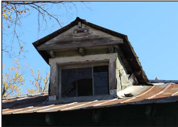
FIGURE 77 . Detail of deteriorated dormer.
