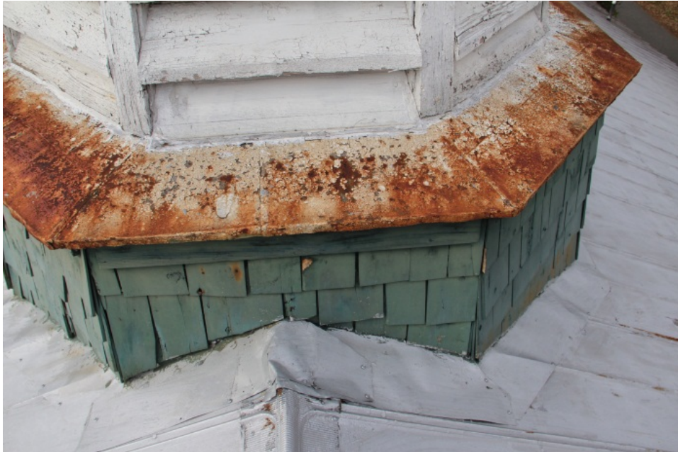
West elevation of cupola base and shelf flashing between base and louvered panels (possibly original) at intersection with primary ridge line. Typical of all base flashing conditions.
