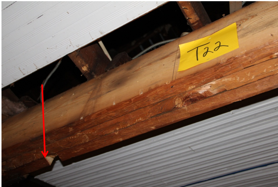
Task 29a. Requested wood ID sample taken at exposed triple built-up beam in ballroom near task 22 marker (see arrow). This beam is part of the Phase 2 expansion of the WCCB ca. 1910.
