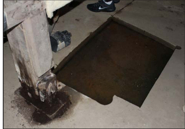
FIGURE 91 Missing section of concrete floor in West Boat Storage Area.
