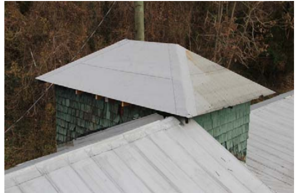
Repaired west slope and older south slope of North Tower hipped roof.
