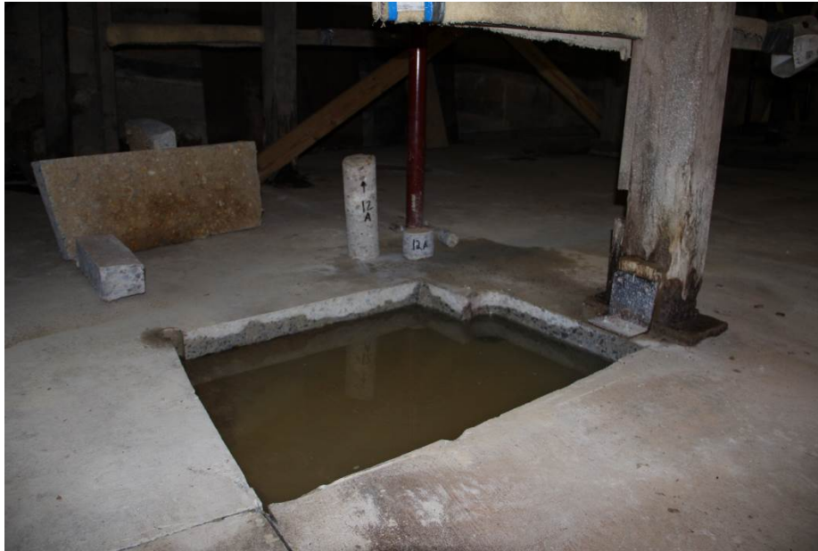
A section of concrete floor saw cut and removed in the West Boat Storage Area (Room 101) to investigate the subfloor and foundation conditions.
