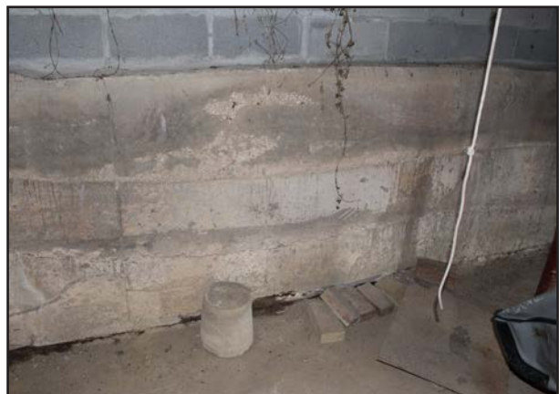
FIGURE 96 Water damage, cracking, and biological growth at north wall of west boat storage area.
