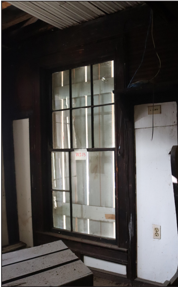
FIGURE 73 Typical double-hung window in Ballroom around the stage. This particular example has missing muntins.
