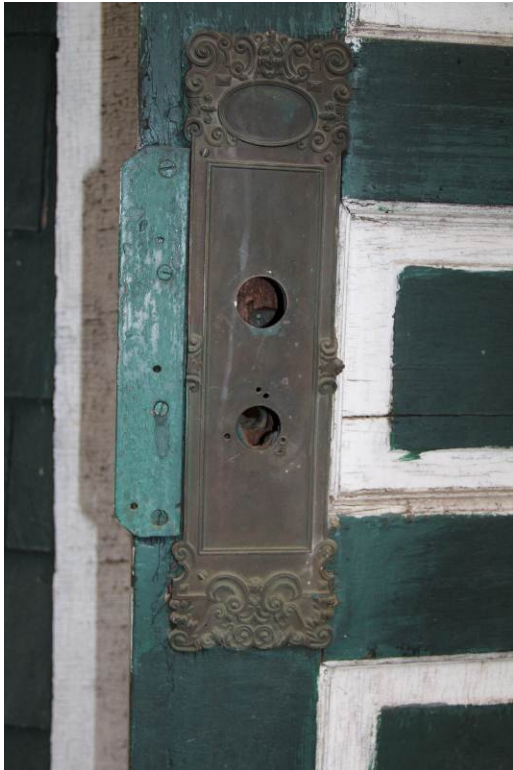
Detail of escutcheon plate at north entrance door. Likely dates to the period of construction after the completion of phase 2 of the main block (ca. 1910). (HPTC photo)
