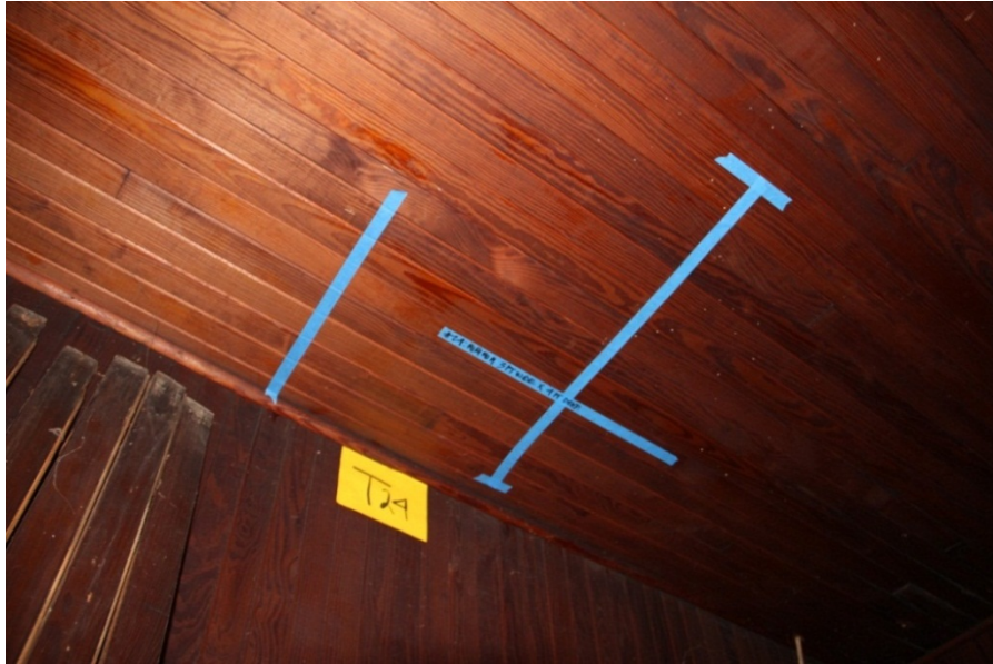
Task 24. Outcome - Ceiling fabric preserved. Ceiling removal above D204; not completed as structure is visible on opposite wall of room.
