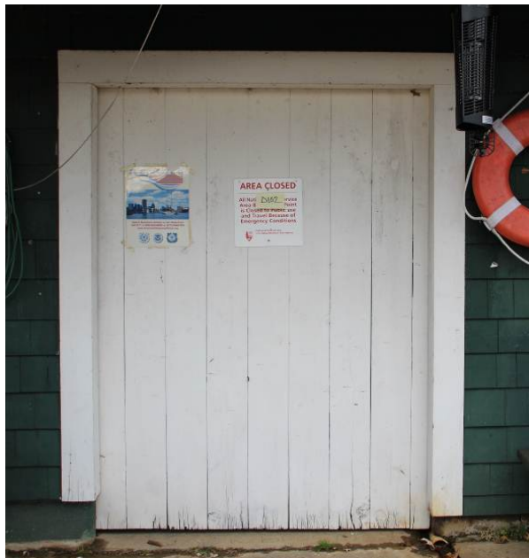
Exterior of swinging door (D102) in the south wall of the West Boat Storage Area (Room 101).
