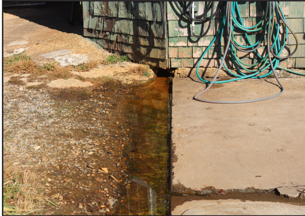
FIGURE 42 Detail of southwest corner of building with drainage trough cut into concrete slab with water discharging from the building.
