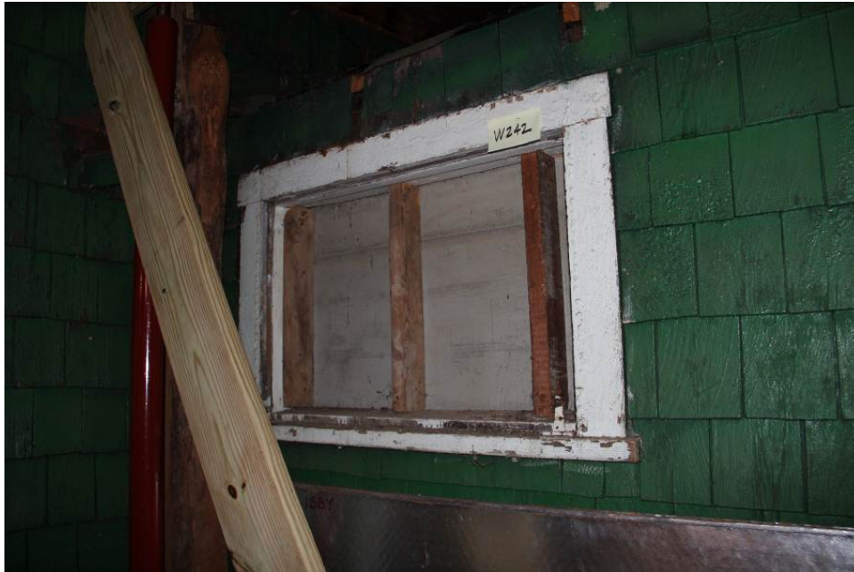
The opening for window W242 is blocked by a shower stall in the Women’s Locker Room (Room 210).
