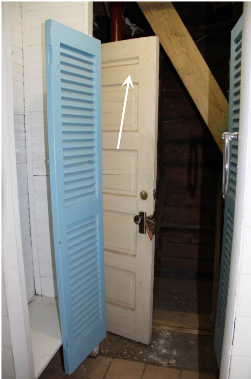
Door (D210) has been modified to fit the opening. Note the small panel at the top of the door (arrow).
