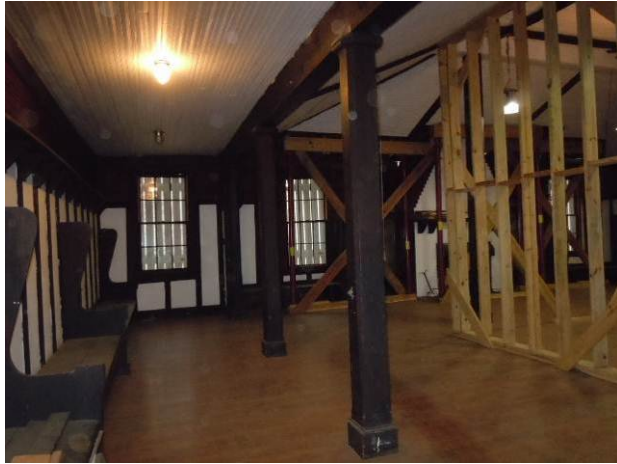
Interior columns which create west gallery space in Ballroom are original to Phase 1 construction. (HPTC photo)
