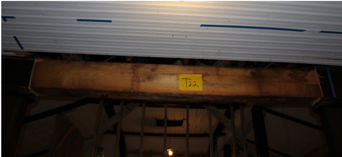
Task 22. Outcome: Skirt boards removed from beam to reveal triple 2X14 beam spanning between posts. NOTE: marks end wall of Phase 1 construction – see historic ballroom image.
