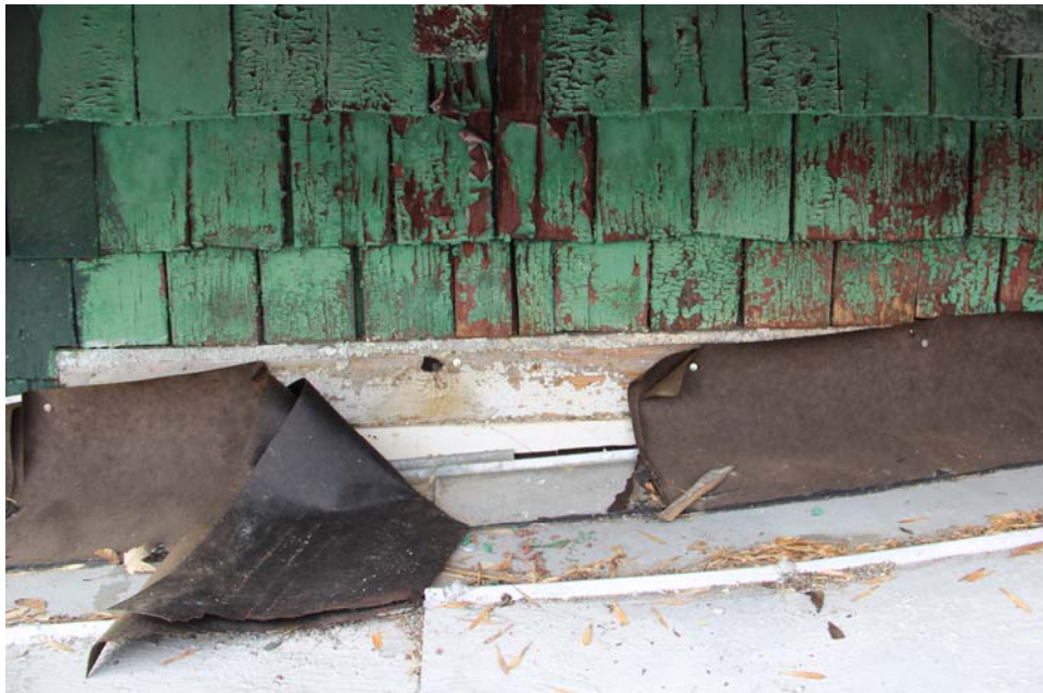
Flashings at roof intersections are failing or non-existent.
