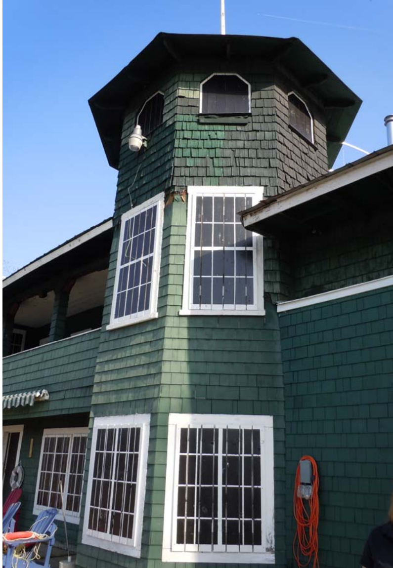
View of Washington Canoe Club exterior in April 2013. Vented window and door covers are seen covering many of the window and door openings.
