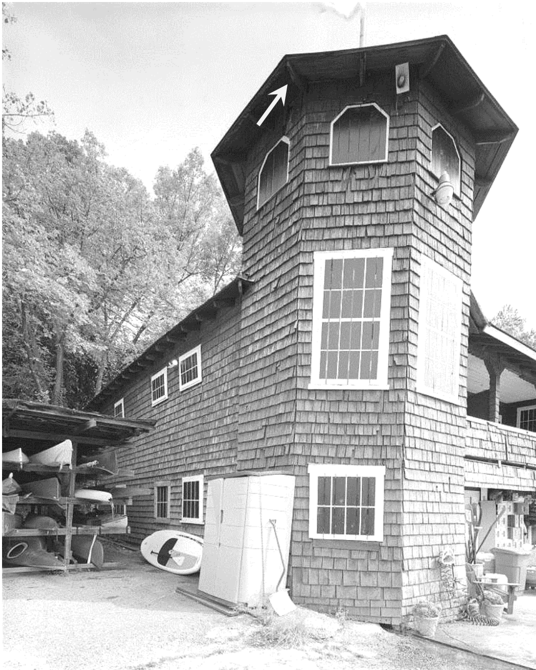
The towers have wide overhangs with exposed rafter tails (arrow). These overhangs are categorized as soffits in this report format. (HABS photo)
