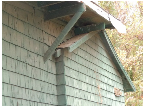
East gable end of Women’s Locker Room roof frame projects beyond wall line of building. Original rafter tails, rake boards and roof sheathing can still be seen.
