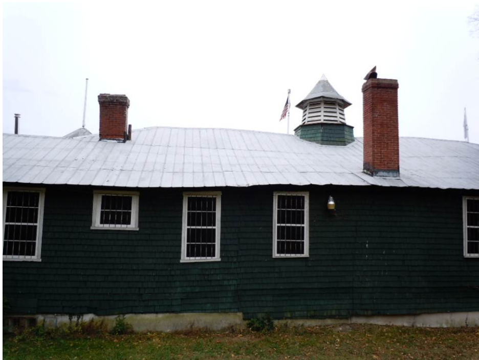
Two red brick chimneys are located on the north slope of the main roof. (HPTC photo)
