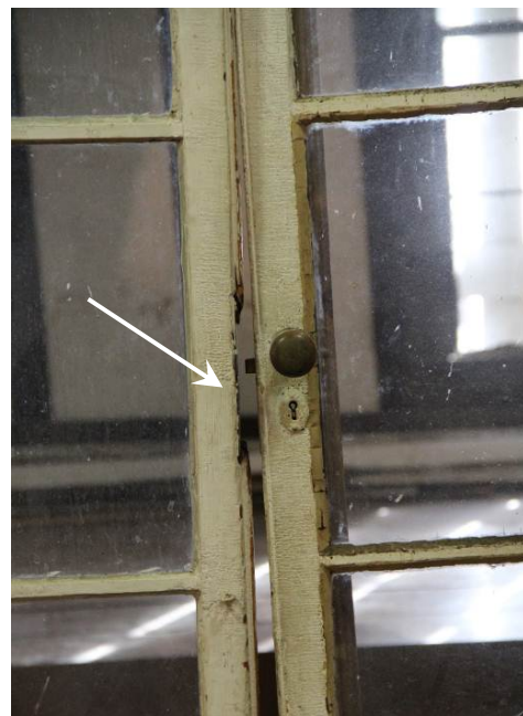
Detail of exterior hardware on double casement windows. Note wood damage on stile (arrow).
