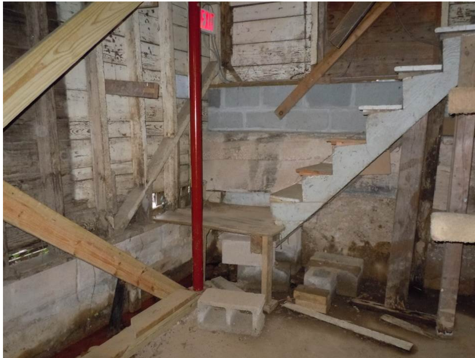
Stairs (ST01) in the northeast corner of West Boat Storage (Room 101) leading to the Men’s Locker Room (Room 203).
