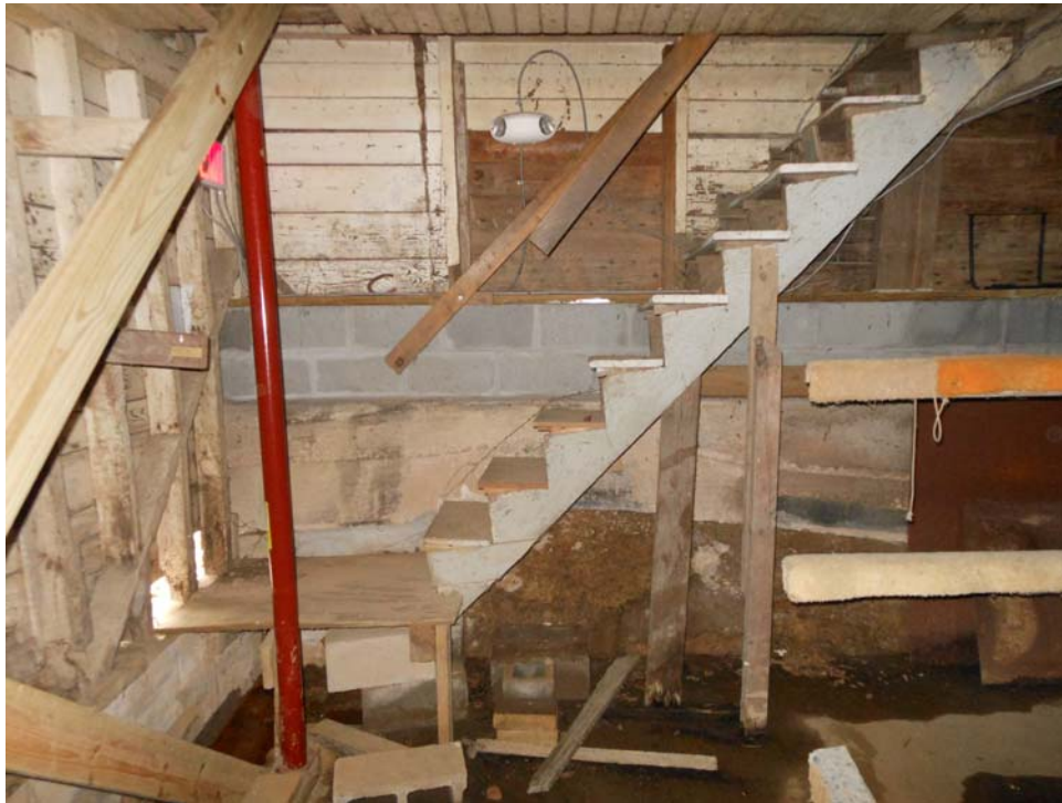
The stairs (ST01) in the northwest corner of the West Boat Storage Area (Room 101) are failing and unsafe.
