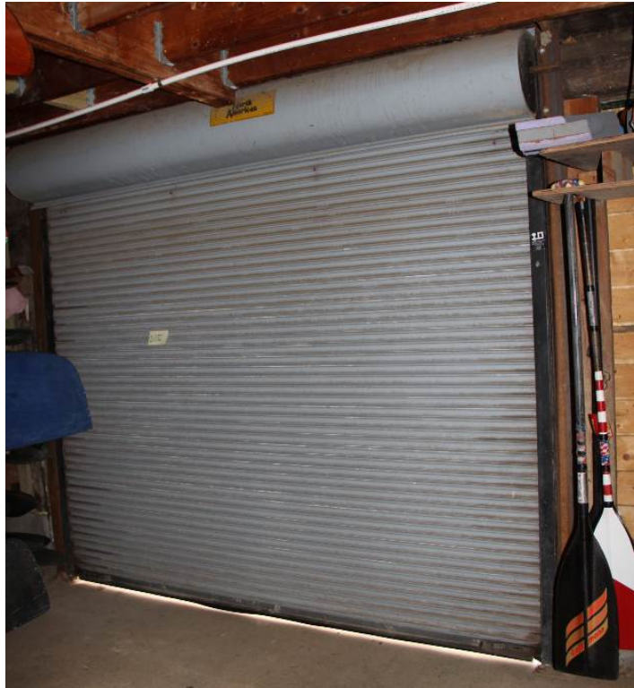
Interior view of typical overhead metal roll-up door in the East Boat Storage Area (Room 106).
