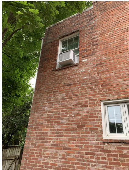
6 REAR VIEW OF NEIGHBORING WALL
