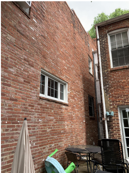
5 REAR VIEW OF NEIGHBORING WALL
