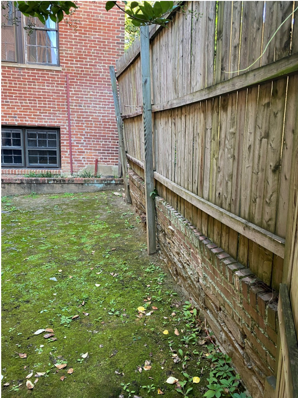
View of Failing brick wall, as viewed from Condo side of the fence
