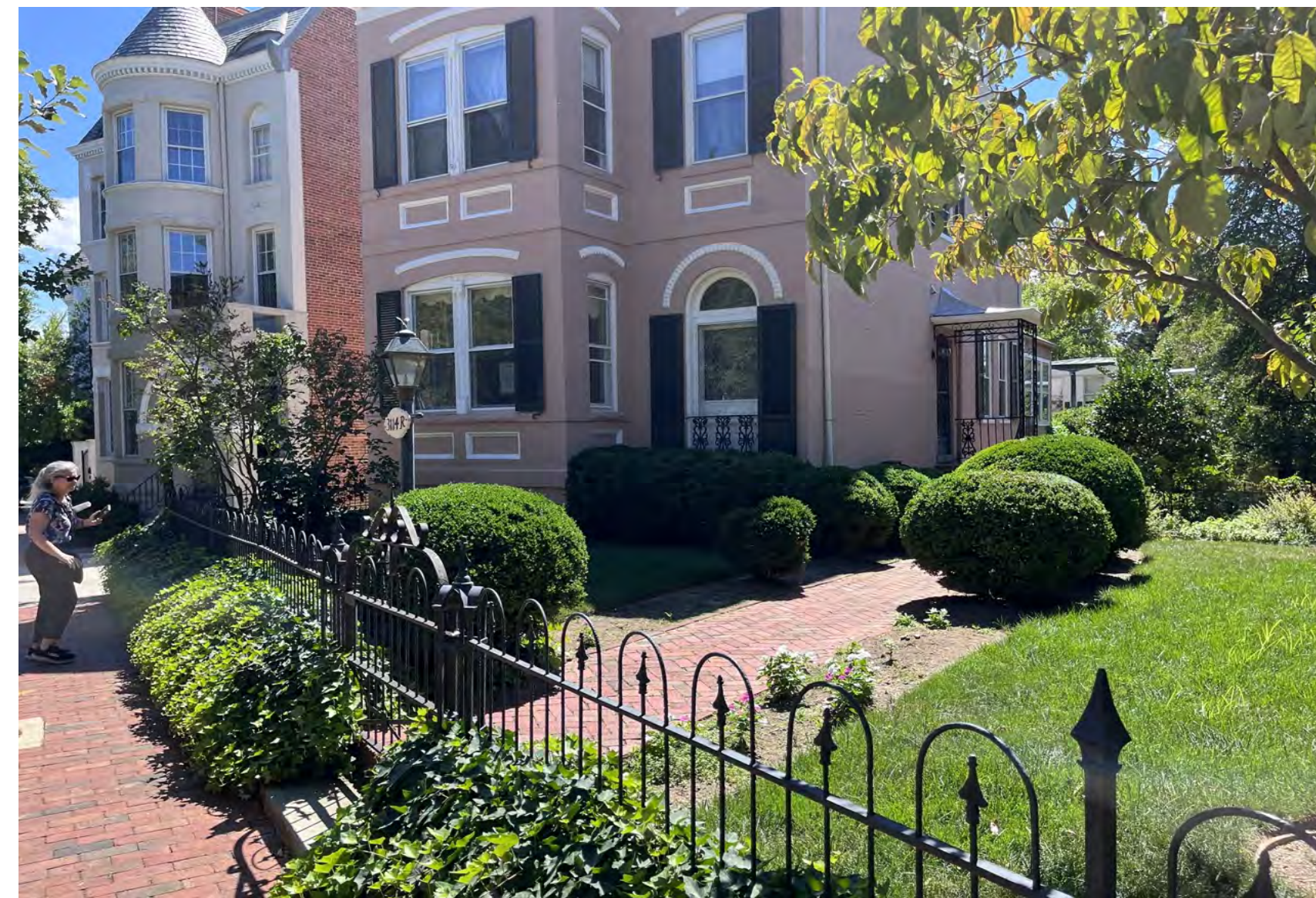
View Looking Towards The House From The Sidewalk (Prior to Start of House Renovation)
