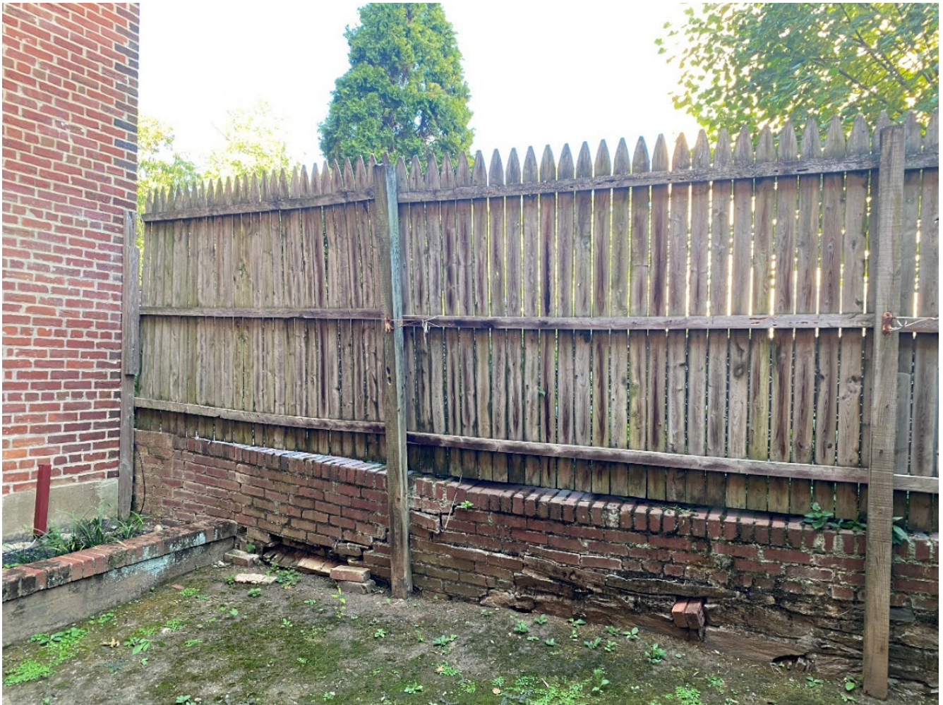
View of Failing brick wall, as viewed from Condo side of the fence
