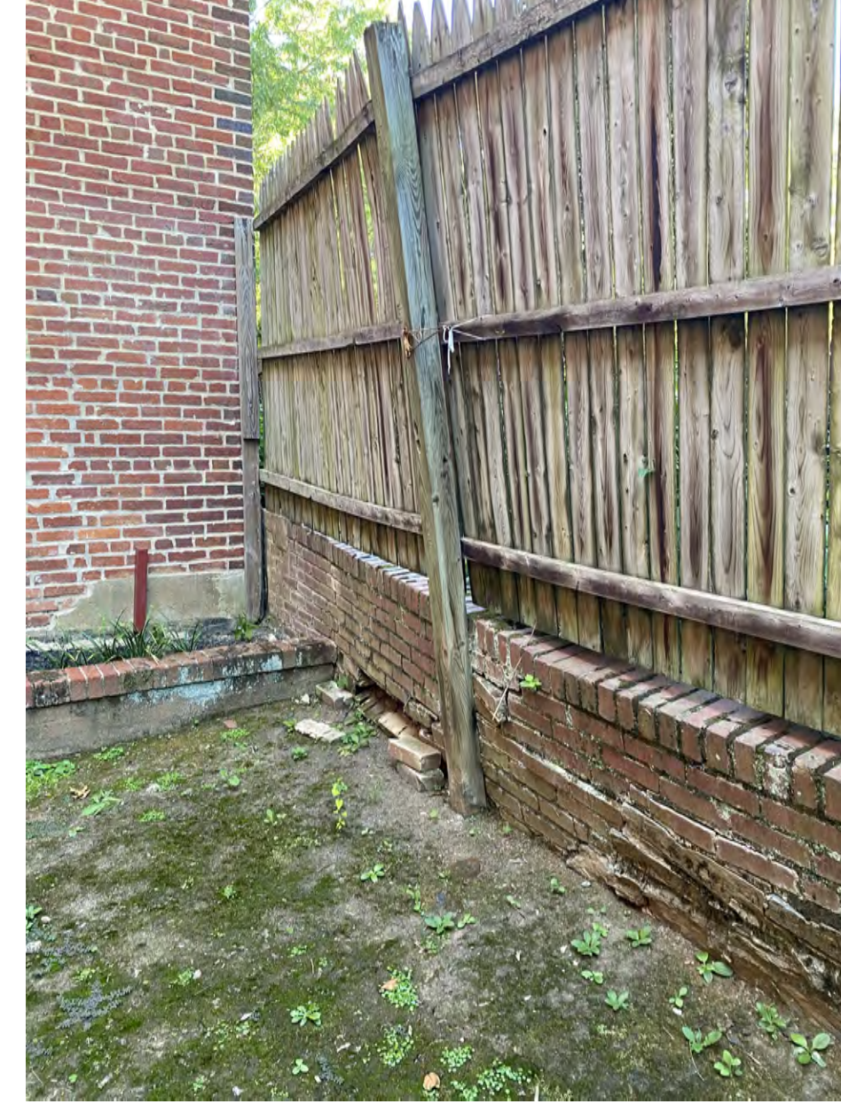
3. Existing failing retaining wall at Condo building
