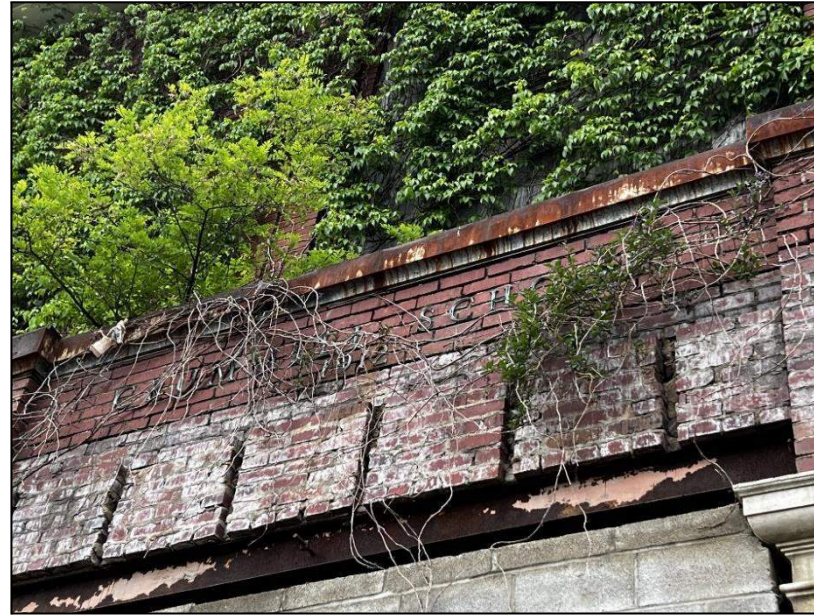
Figure 2: South entrance, missing cornice. Note lettering.
